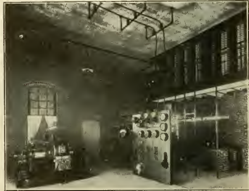
Ben-Hur Route—Interior of Substation.
