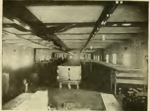
Ventilating New York Central Power Stations—Battery Room, Yonkers.
