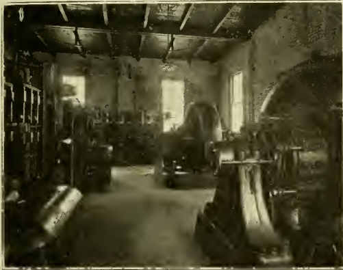
Chicago & Southern—Interior Blue Island Substation.
