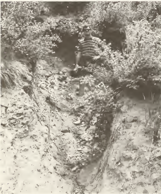
Figure 11. — Large gully in slope, Watershed No. 1, Pine Creek study area, Boise National Forest, Idaho. Gully was formed by subsurface flow emerging at cut face followed by piping and "spring sapping," which triggered localized slope failure. (Photo taken July 1977.)
