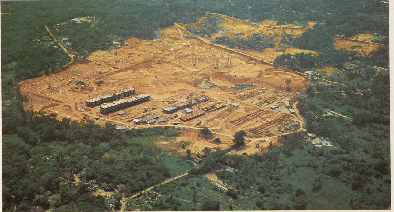
The first group of blocks of flats under construction at Ang Mo Kio New Town. ▲ A new L-shaped block with three-room Improved flats at Toa Payoh New Town. ▼
