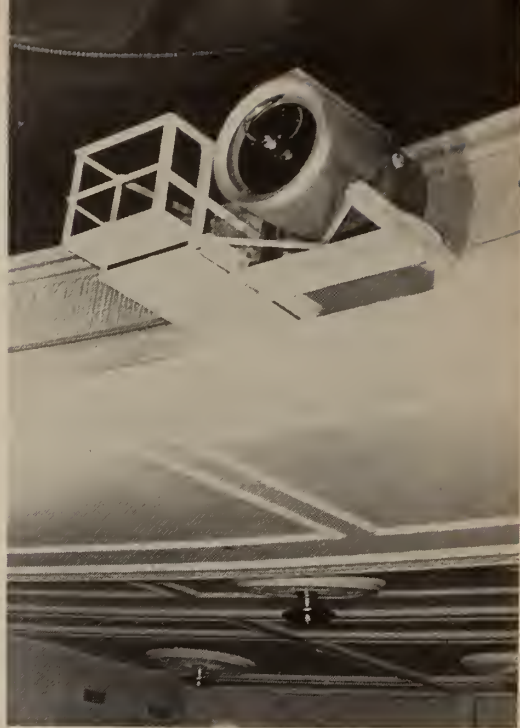
RCA theater television projector mounted on front of theater balcony.
