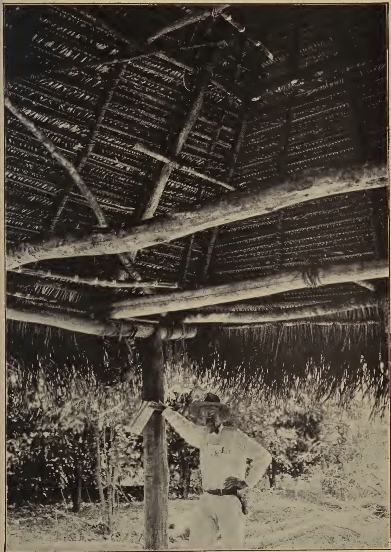
Nails are but little used in Mexico, either by skilled carpenters or Indian hut builders. Poles for scaffoldings or the frames of houses in the jungle are tied together with ropes or withes.
