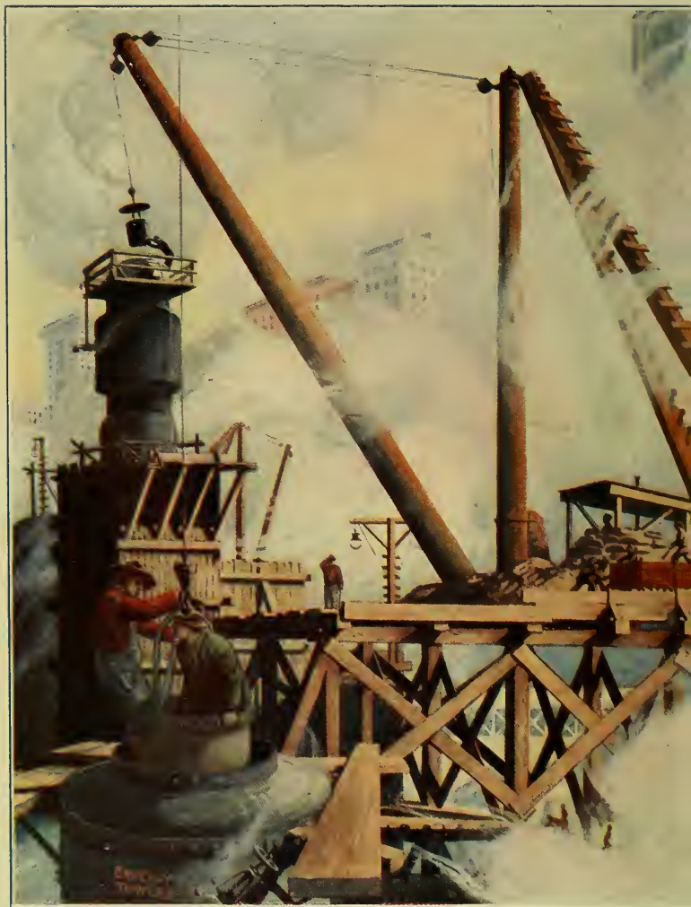
"A CONFUSION OF DERRICKS, CONCRETE MIXING MACHINES, BUCKET ELEVATORS, ENORMOUS WOODEN BOXES, AND CURIOUS CYLINDRICAL OBJECTS. . . ."
