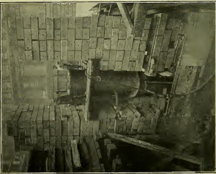
CAISSON WEIGHTED WITH IRON BLOCKS TO FORCE IT DOWN. BETWEEN THE PILES OF BLOCKS IS THE AIR-LOCK.
