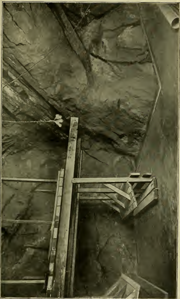
THE DYNAMITE CHAMBER. NOTE THE COVERED SHELVES ON WHICH THE POWDER IS STORED.
