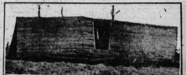
A negro farm tenant, his wife and their child, were in this house when a tornado picked it up, carried it 12 feet and dropped it on its roof in Wake County, N. C. The occupants escaped unhurt.
