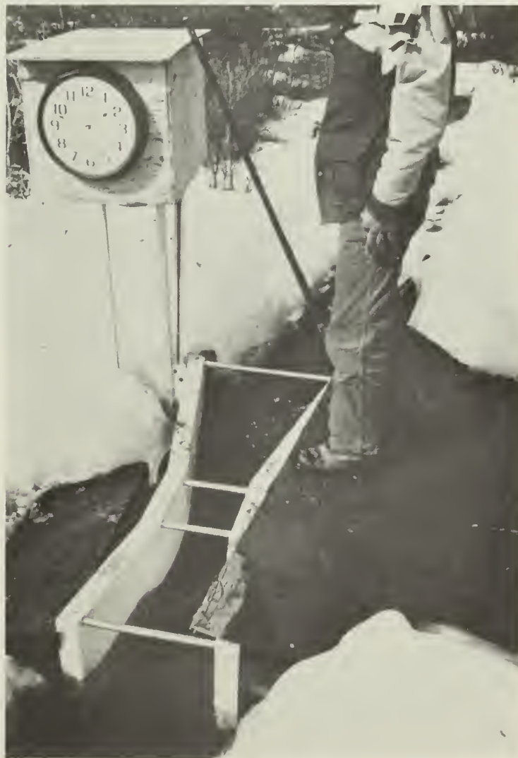
Figure 2.—Parshall flume in C-2 channel; ice surrounds flume in late April. Clock was added for time-lapse photography at the site.
