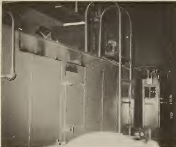
Figure 15. Typical oven used to elevate the temperature of products by indirect heating. Note the single burner in the heat exchanger on top of the oven.
