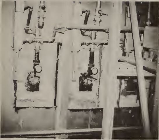
Figure 9. Section of small high temperature tunnel kiln. This photograph shows three of the burners in this section of the kiln.
