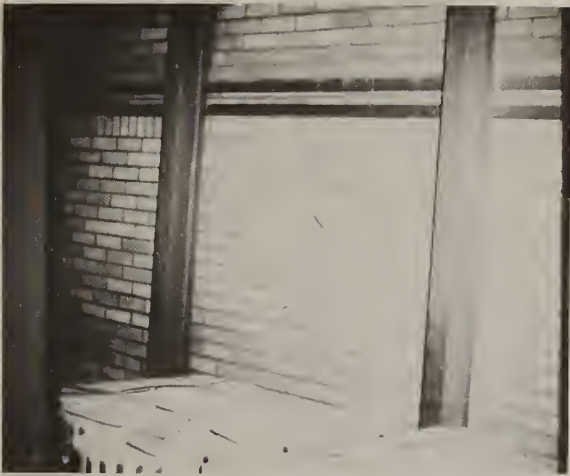
Figure 5. Outer wall of the exit of a small tunnel kiln used to fire building brick. Inner walls and ceiling constructed of refractory brick.
