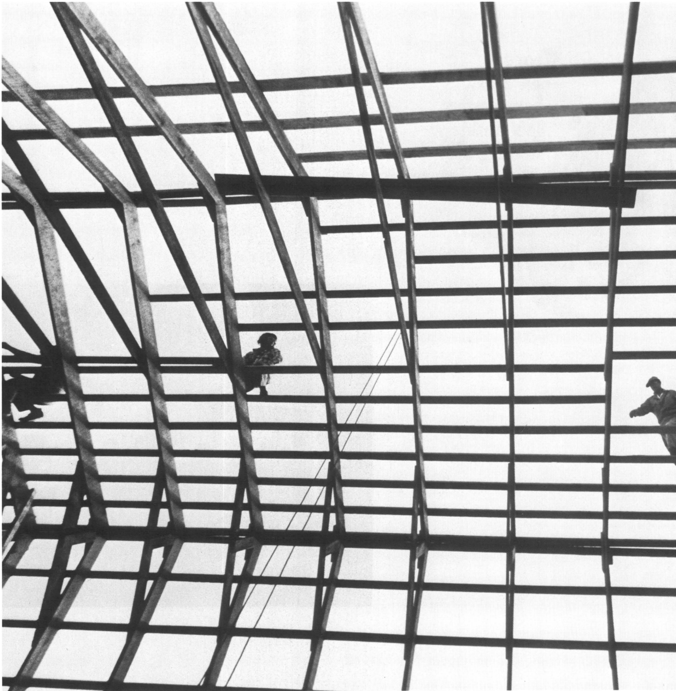
When fire destroyed Ron and Jane Nipple's dairy barn, near Millerstown, Pa., neighbors set aside several consecutive Saturdays to rebuild their barn. The sturdy oak timbers were home-grown.
