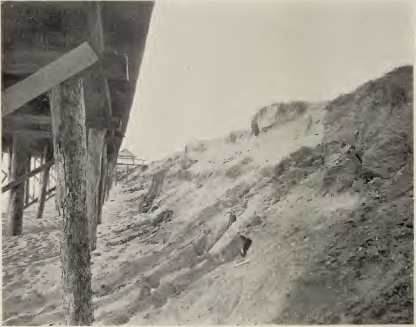
Washout on the Beach, near Ross's, after the September High Tides.
