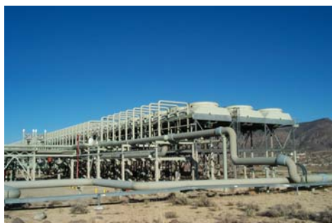
Power plants include a variety of infrastructure, including cooling towers.
