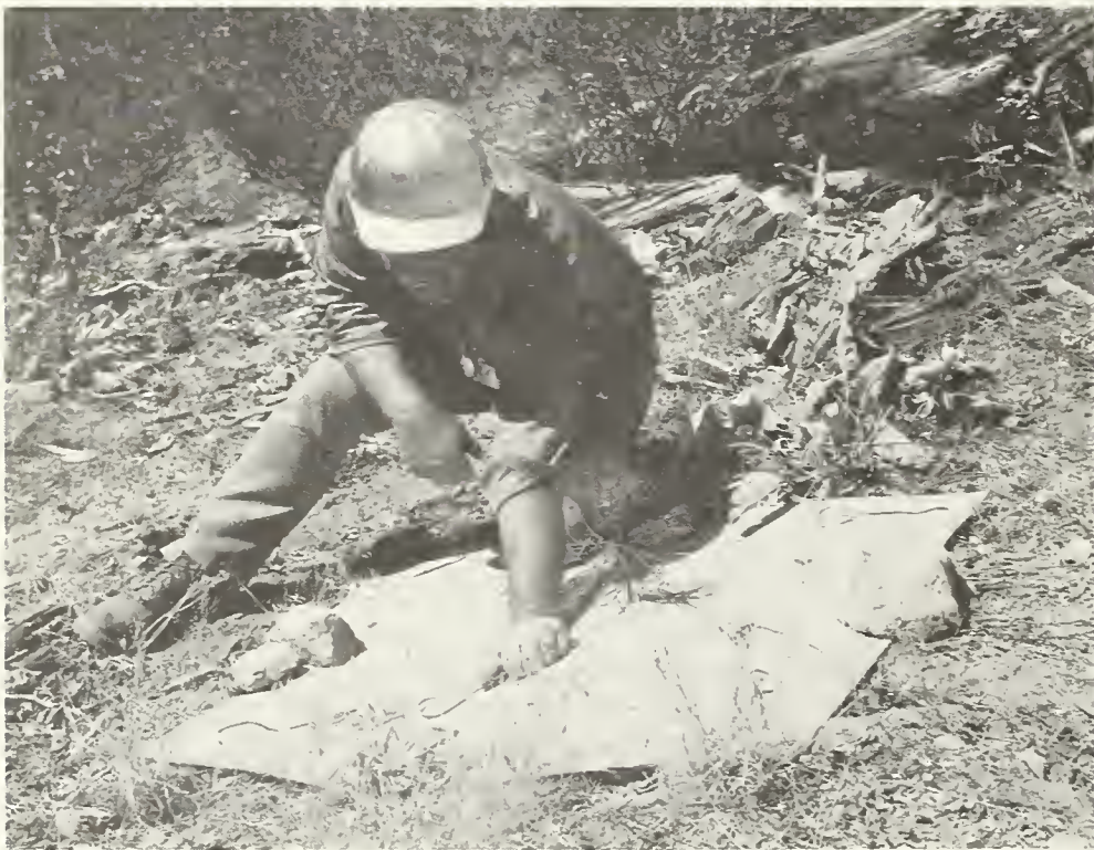
Figure 5.--Glass fiber blanket serves as mulch and is held in place with wire pins.
