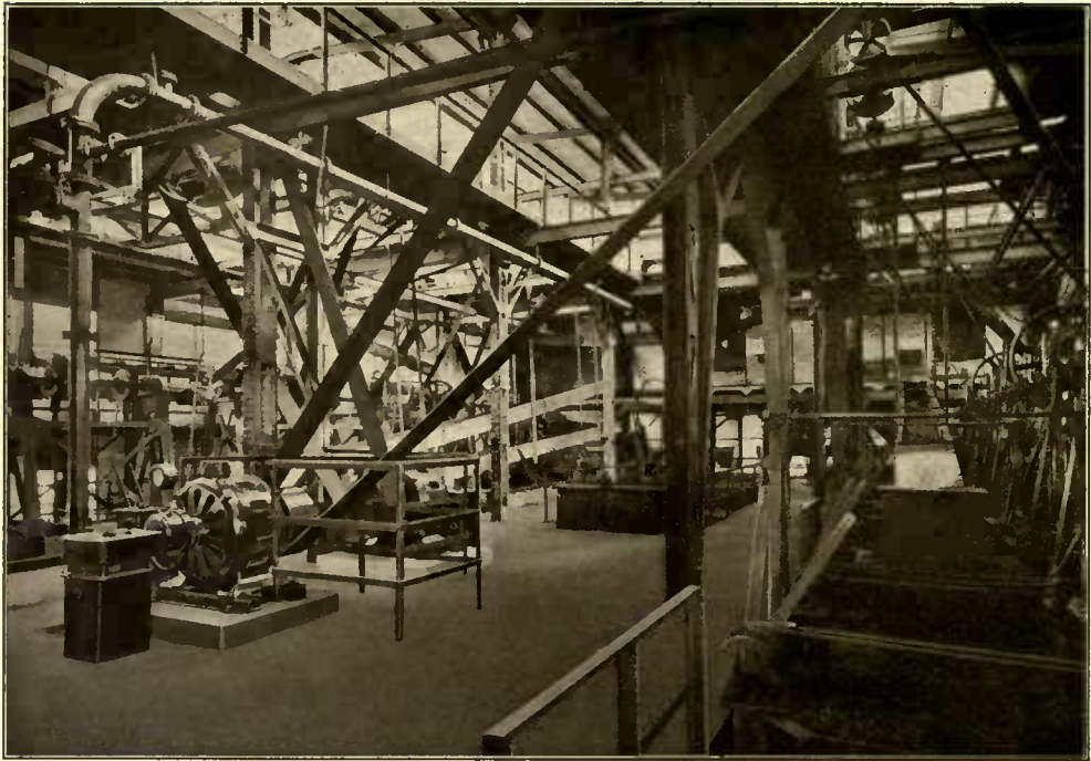
Fig. 140 Coal Washery of the "Bergmannsglück" Mine, Buer (Germany). Motor with starter and control pillar.
