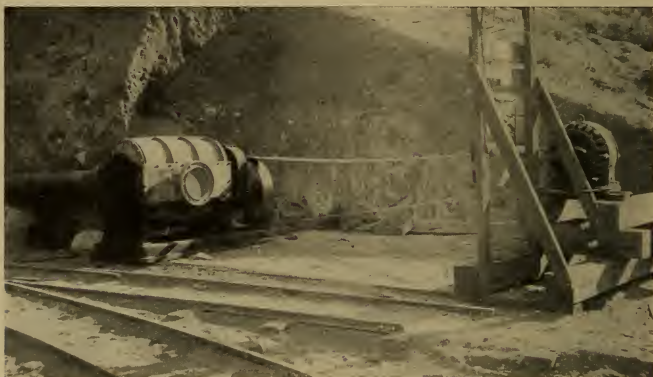
FIG. 26. Ventilating blower used on Los Angeles Aqueduct.
