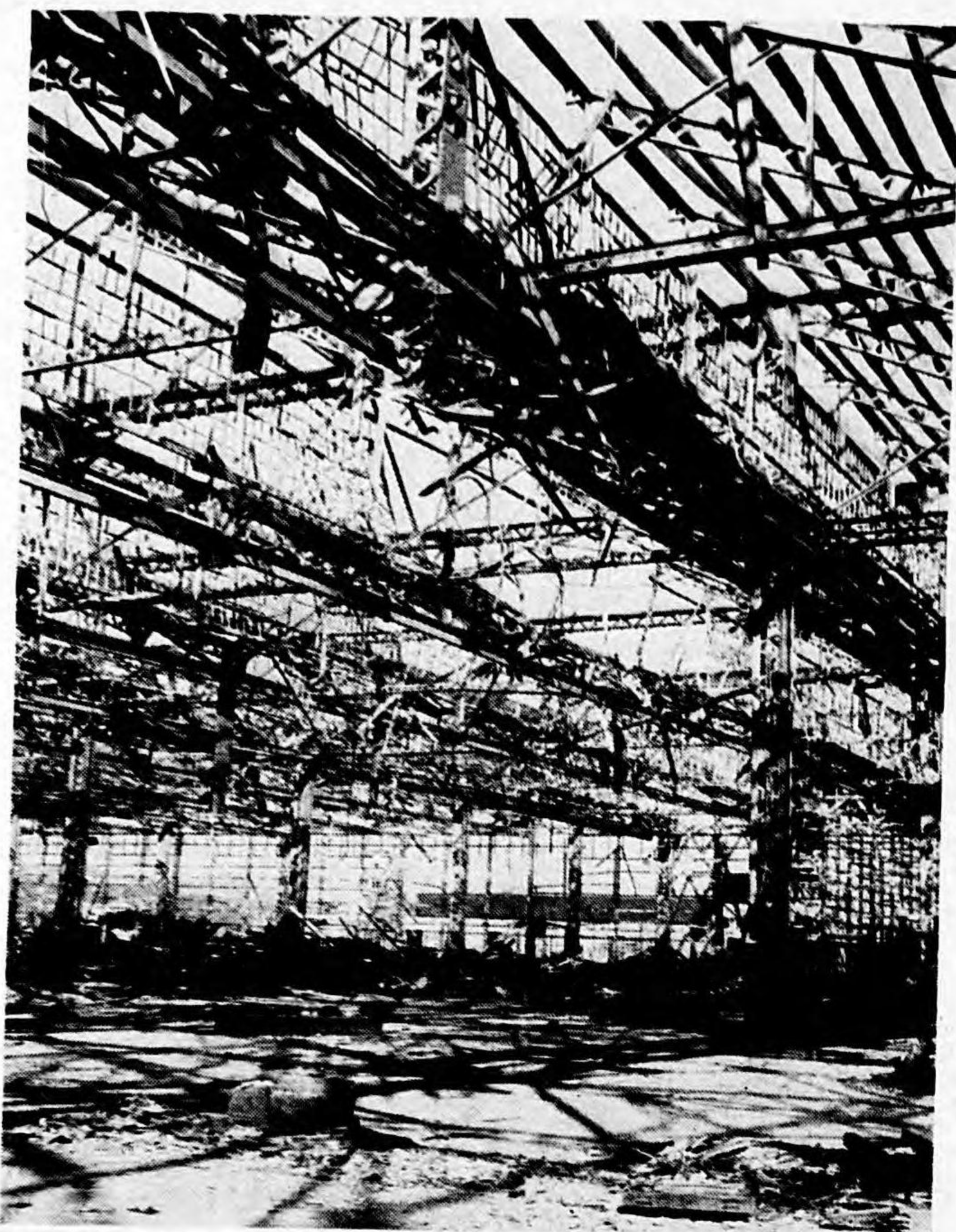
Photo 12.—Building 3, Bomb 17; column destroyed; view of damage and debris.
