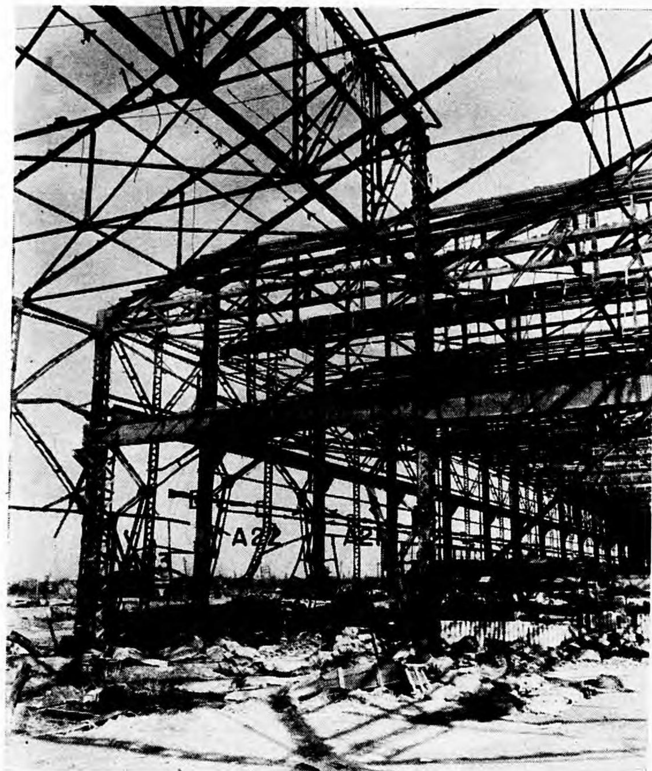
Photo 14.—Building 304; damage to crane girder looking NNE.
