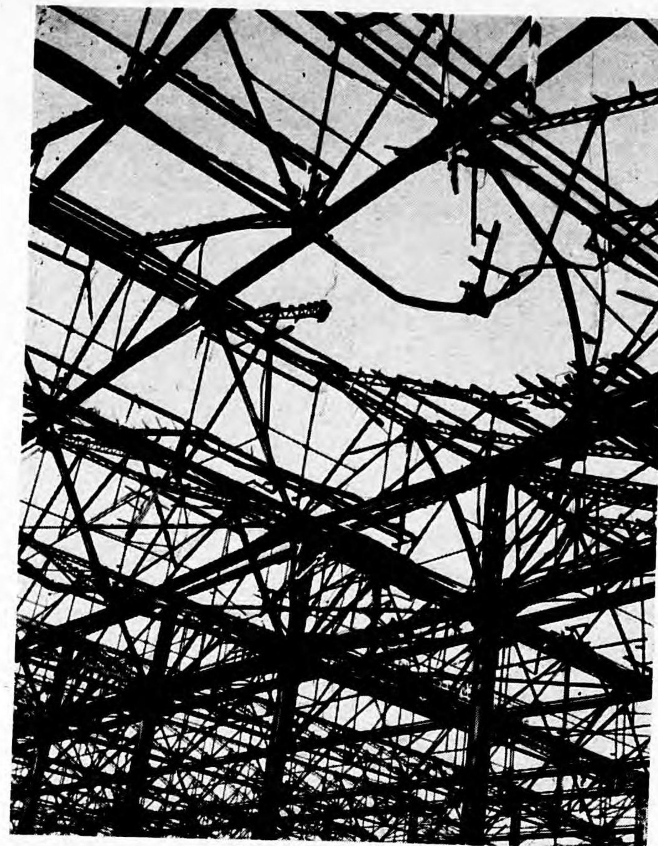
Photo 5.—Building 2, Bomb 6; damage to roof steel; bent hoist runway.
