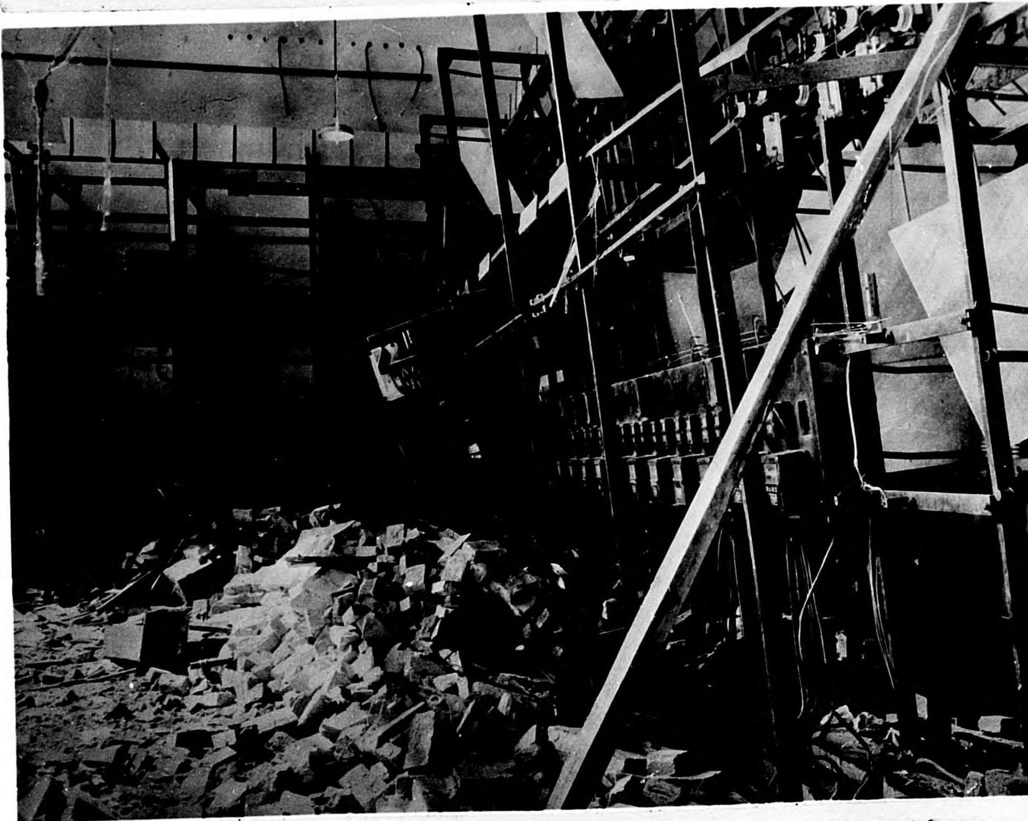
Photo 125. Nagasaki, 5,400 feet from GZ, Zenza Substation. Controls, 3.5-kv busses and oil-circuit breakers.
