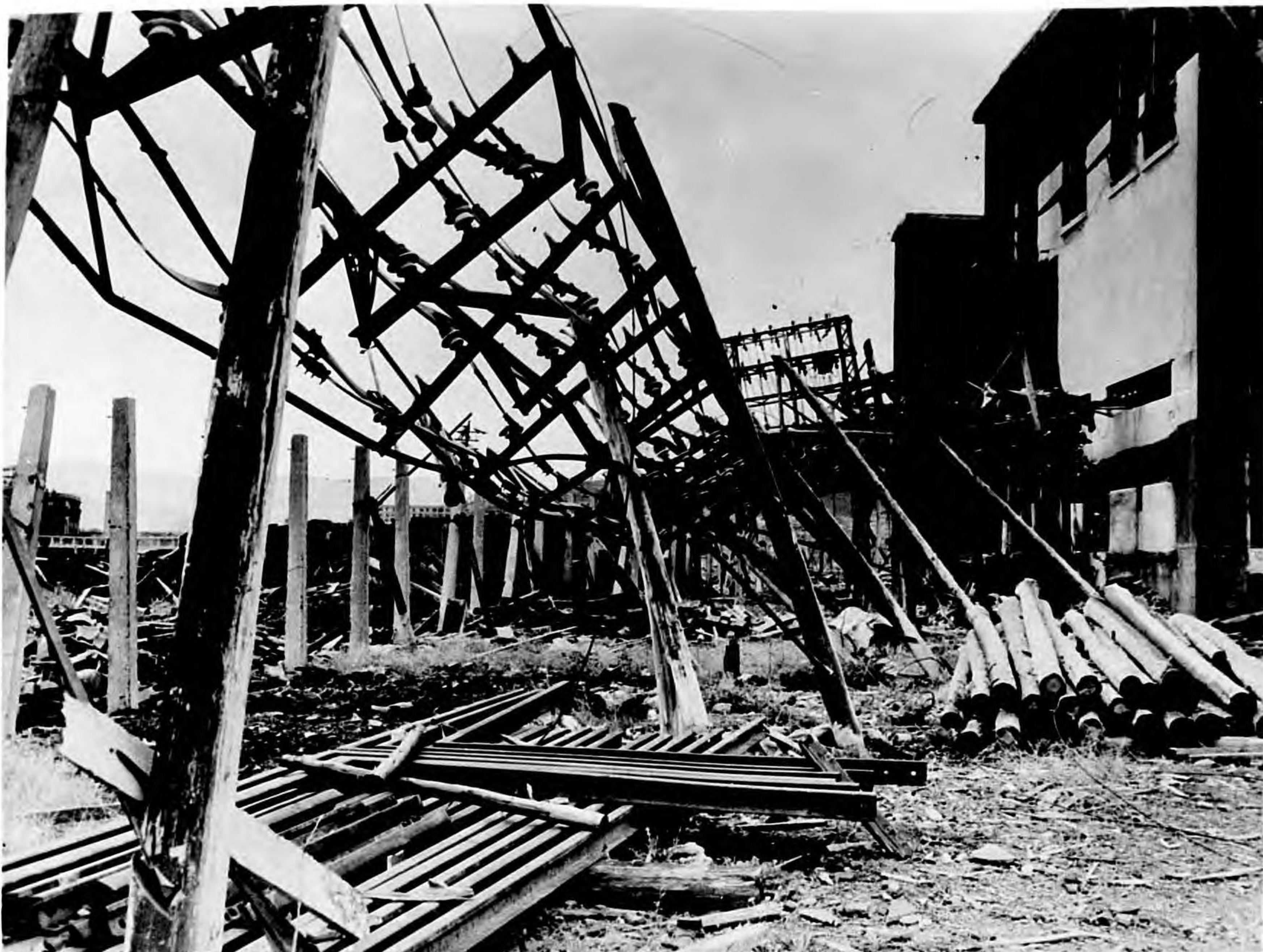
Photo 122. Nagasaki, 3,600 feet from GZ, Takenokube Substation. Damage to three-circuit copper bus structure. Flash burns on poles.
