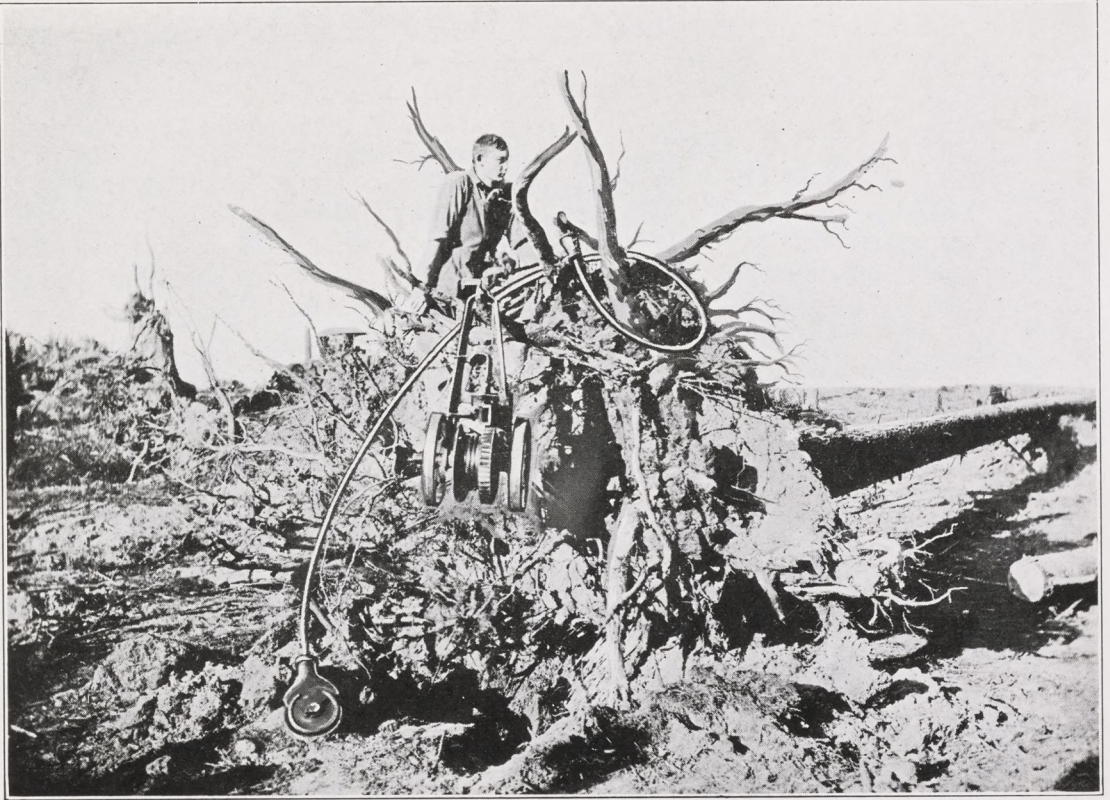
This 32-inch pine tree was pulled clear of the ground by a Bull Dog Hand-Power Machine. The 18-year-old lad in the picture operated the machine. The power pulley and cable were attached about eight feet above the ground
