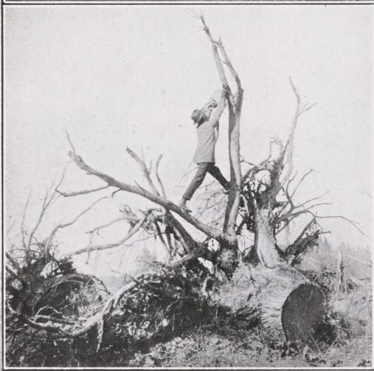
Another photograph showing how thorough the 90-ton Bull Dog Horse-Power Machine is in removing the roots of stumps. The roots of this immense fir stump had a spread of over 32 feet. By comparing them with the man in the picture you will get a good idea of their size
