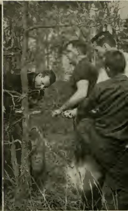
Building a barbed wire fence around the unwed mother's home in Durham.
