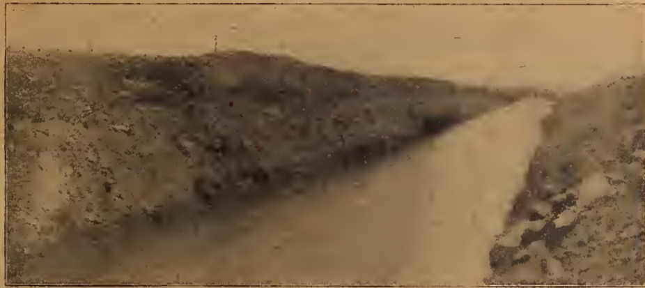
Main canal of the Laramie-Poudre Irrigation Company now being constructed. Ditch twenty-two feet wide at the bottom. Takes water from the Laramie River across to the North Poudre and down it to the canal heads
