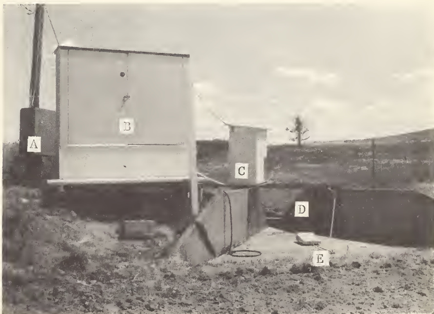
Figure 13.--Runoff measuring and sampling installation, looking downhill from experimental watershed: A, switchbox for electric power; B, shelter for refrigerator, sampler pump, and controls; C, shelter for water-stage recorder, and stilling well for float and mercury on-off switch; D, runoff rate measuring flume; E, intake sampling tube; F, purge discharge line from pump.
