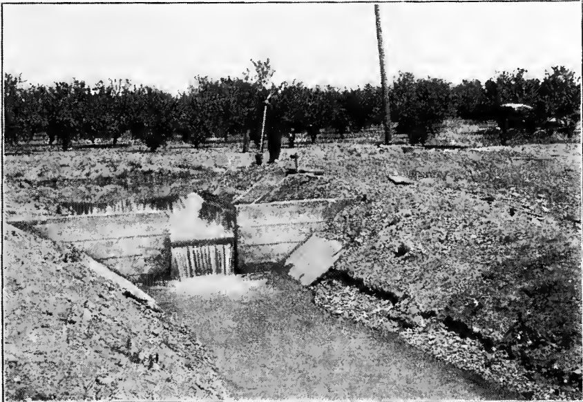
FIG. B.—Concrete box and drop on distributory in place of earlier form of wooden construction. Orland Project, Cal.
