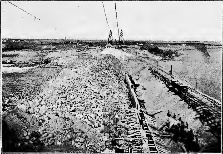
FIG. A.—Earth and rockfill dam under construction, with low concrete core wall, gravel and earth is being dumped on upper side with loose rock below, Minidoka, Idaho.
