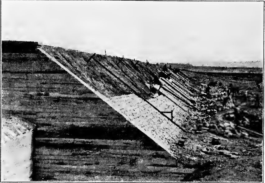
FIG. C.—Paving on water side of earth embankment. Belle Fourche River, So. Dak.
