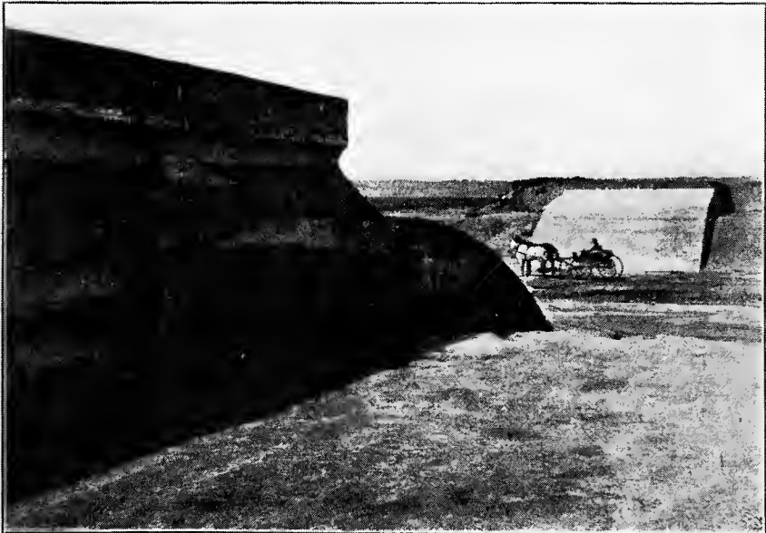
FIG. B.—Concrete inverted siphon carrying water of main canal under side drainage line instead of over it. North Platte Project, Wyo.-Nebr. (Facing Page 88)
