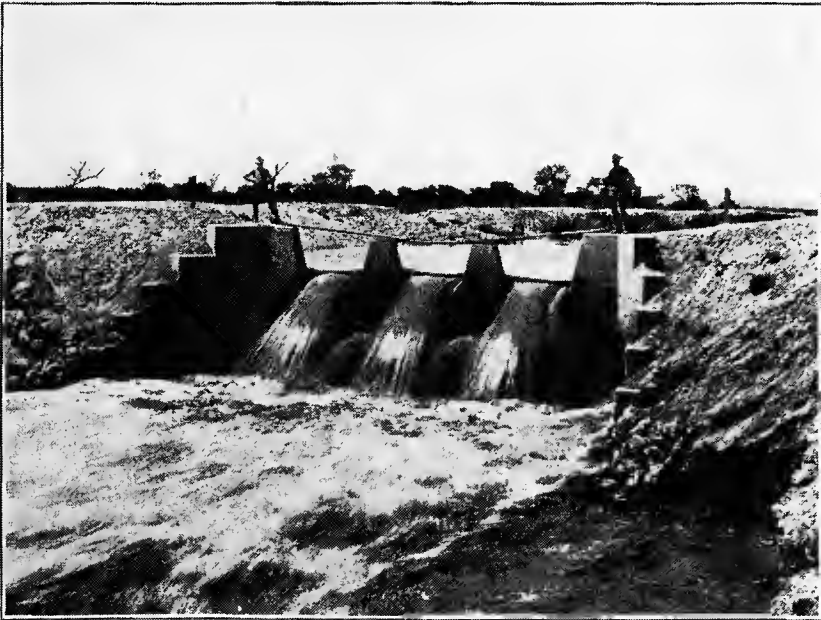
FIG. B.—Notched check and drop with projecting lip beneath each notch to diffuse and break the force of the falling water. Rio Grande Project, N. Mex.
