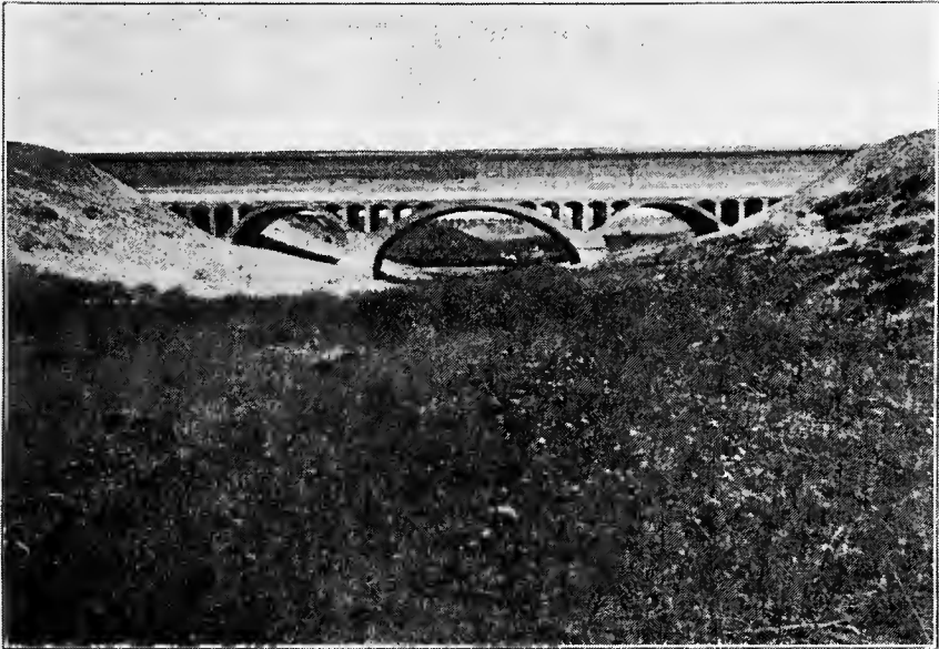
FIG. A.—Concrete flume carrying water of main canal across side drainage lines. North Platte Project, Wyo.-Nebr.
