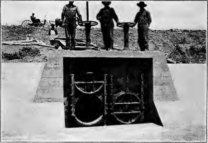
FIG. C.—Cast-iron valves on distributing systems instead of the usual wooden gates. Uncompahgre Project, Colo.
