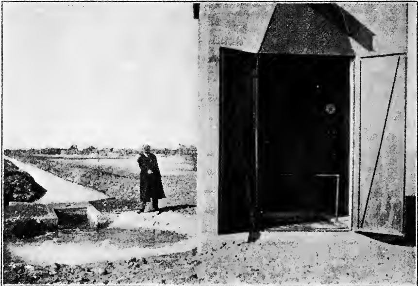
FIG. D.—Electrically operated centrifugal pumps delivering water to laterals on Gila River Indian Reservation, Ariz.
