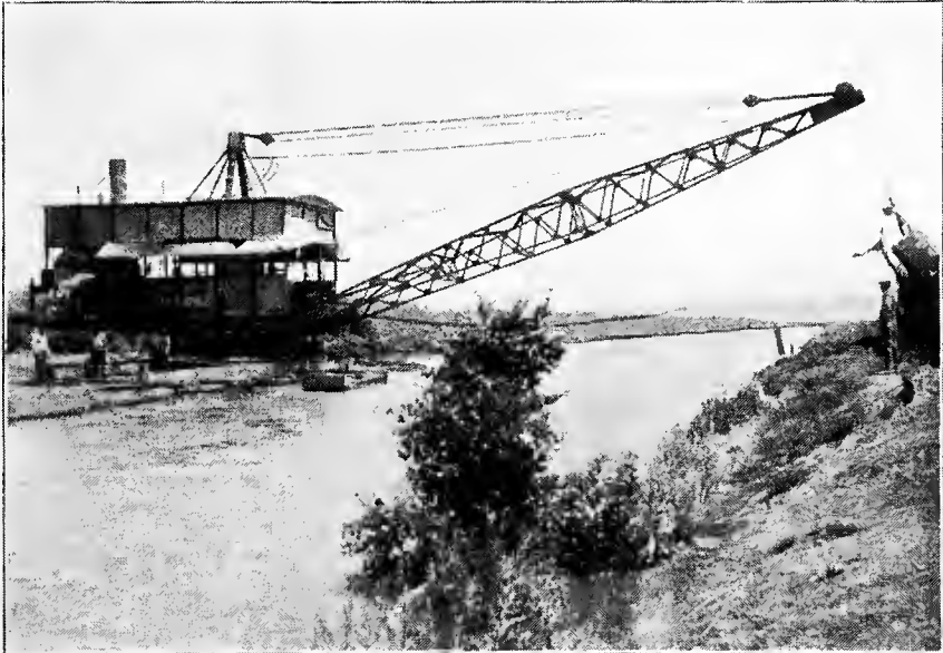
FIG. B.—Enlarging canal by use of excavator with drag-line working from one side of canal. Salt River Project, Ariz.
