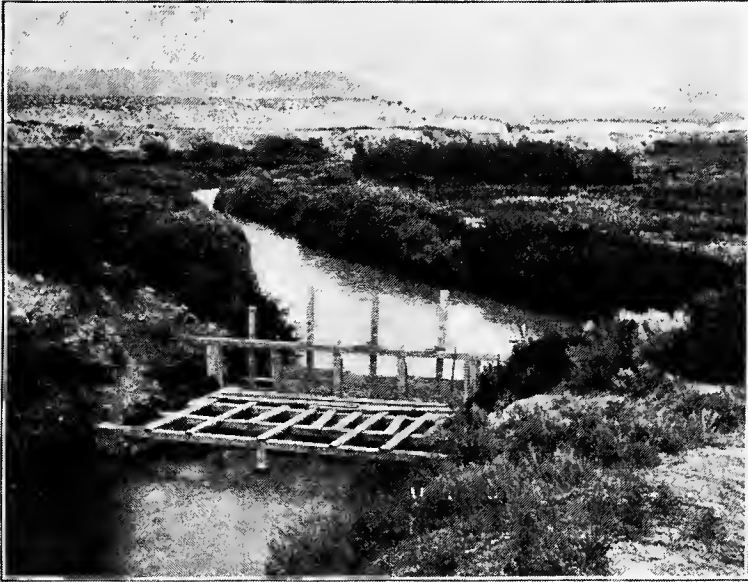
FIG. A.—Wooden headgates, typical of those usually built for the earlier canals. Jordan and Salt Lake City Canal, Utah.
