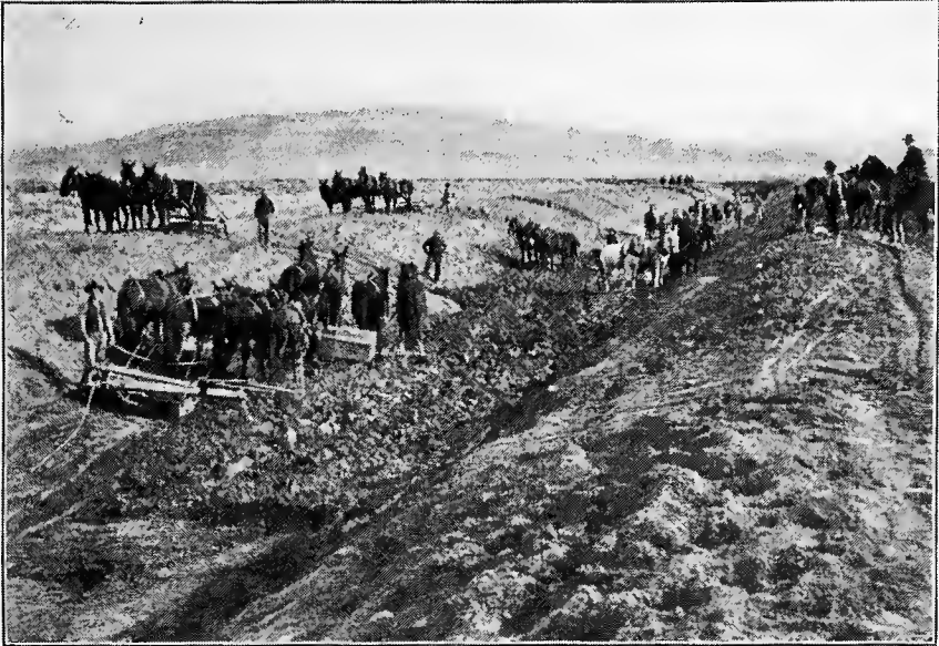
FIG. A.—Constructing canal in earth by means of four-horse Fresno scrapers. Minidoka Project, Idaho.
