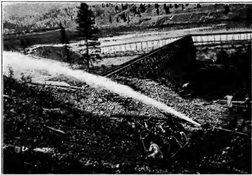
FIG. C.—Hydraulic construction of earth dam, giant in foreground washing earth and small rocks into flumes supported on trestles and conveying materials to site of dam. Okanogan Project, Wash.
