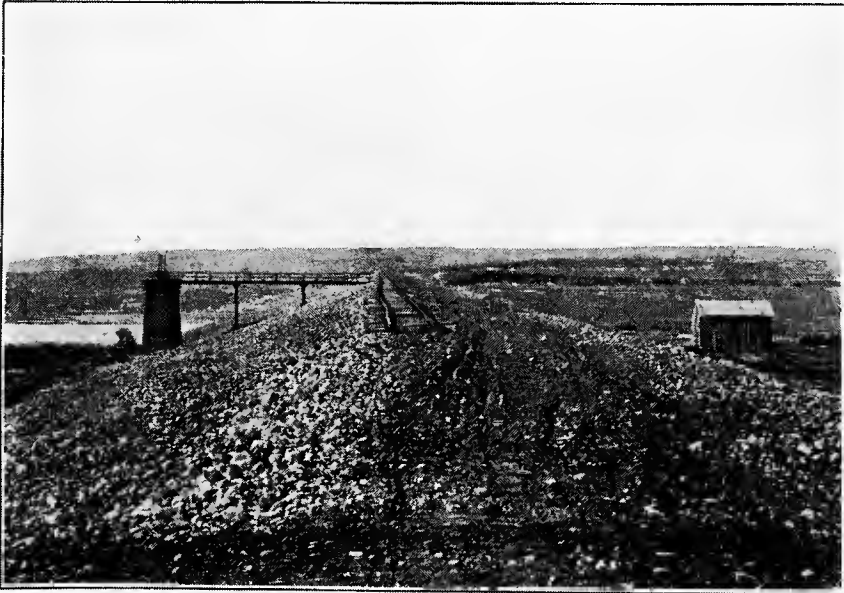
FIG. B.—Earth dam partly protected by heavy gravel on water side. Boise Project, Idaho.
