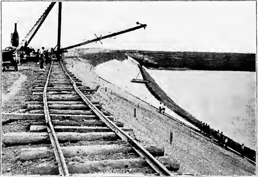
FIG. D.—Concrete block protection against wave action on earth dam. Belle Fourche Project, So. Dak.
