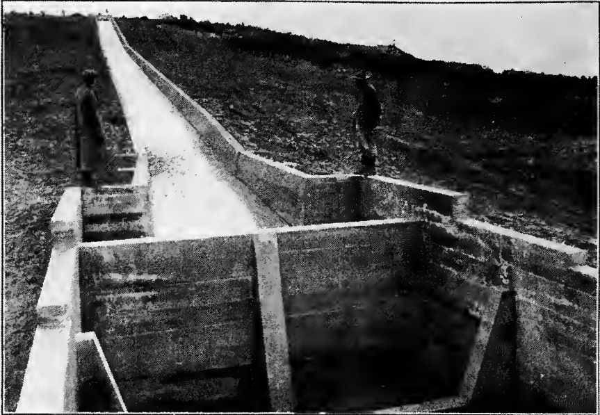
FIG. C.—Concrete chute, built instead of a series of drops, and terminating in a water cushion with concrete baffle board. Boise Project, Idaho.
