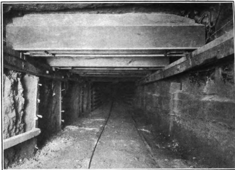
1. TROUGH BARRIER IN PLACE IN A MINE ENTRY.
