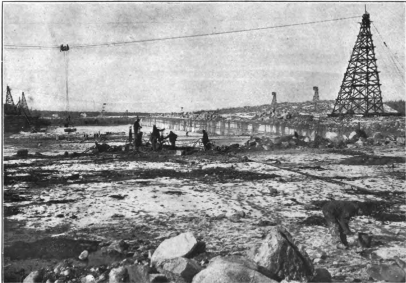
2. ROCK EXCAVATION IN THE WEST NEEBISH CHANNEL, LAKE HURON. WORK CARRIED ON WITHIN COFFERDAMS.
