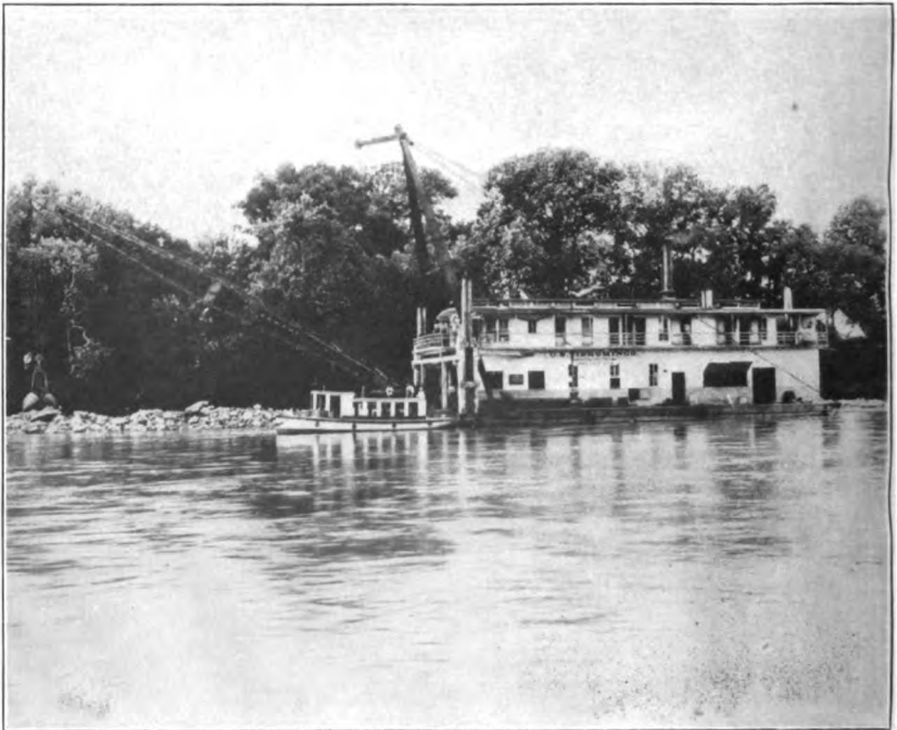
2. CRANE BOAT ON BIG BEND SHOAL, TENNESSEE RIVER. THE GRAPPLE BUCKET HANDLES THE LOOSENED ROCK, PREVIOUSLY BLASTED, IN ONE MOVEMENT FROM CHANNEL TO TRAINING WALL.
