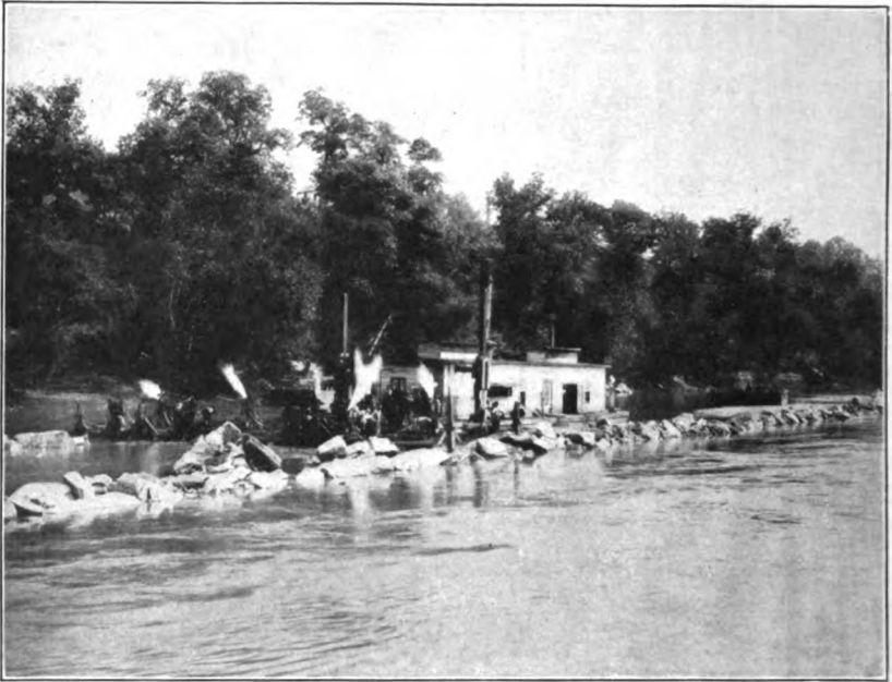
1. ROCK EXCAVATION ON THE TENNESSEE RIVER. SPECIALLY DESIGNED DRILL RAFT BORING PREPARATORY TO BLASTING.
