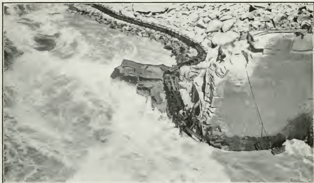
Temporary Fishway through which several thousand salmon passed up.
