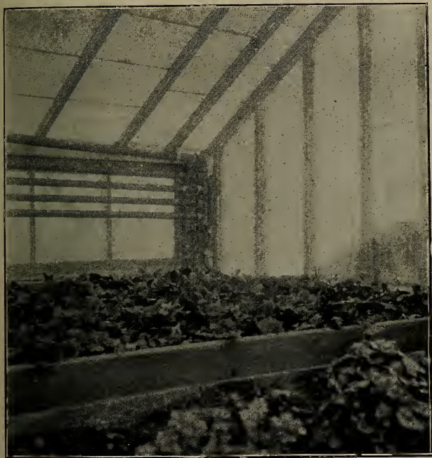
17.—Interior of house, showing method of connecting flow pipe with four returns.
