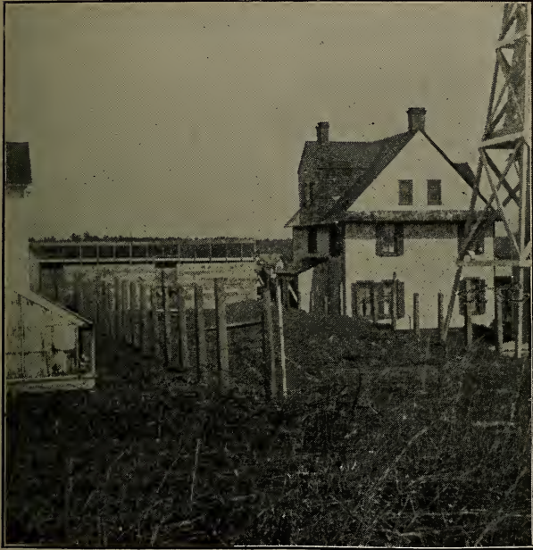
22.—House twenty-four feet wide; posts set and shed at north end built first.
