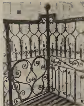
Detail of original wrought iron balcony over door of Congress Hall, Philadelphia
