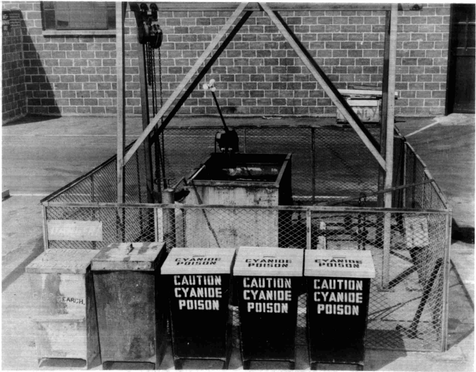
FIGURE 5, IMPROVED CYANIDE DESTRUCTION SYSTEM INCORPORATING SAFEGUARDS SURROUNDING TANK AND BETTER HANDLING EQUIPMENT FOR WASTE CYANIDES
