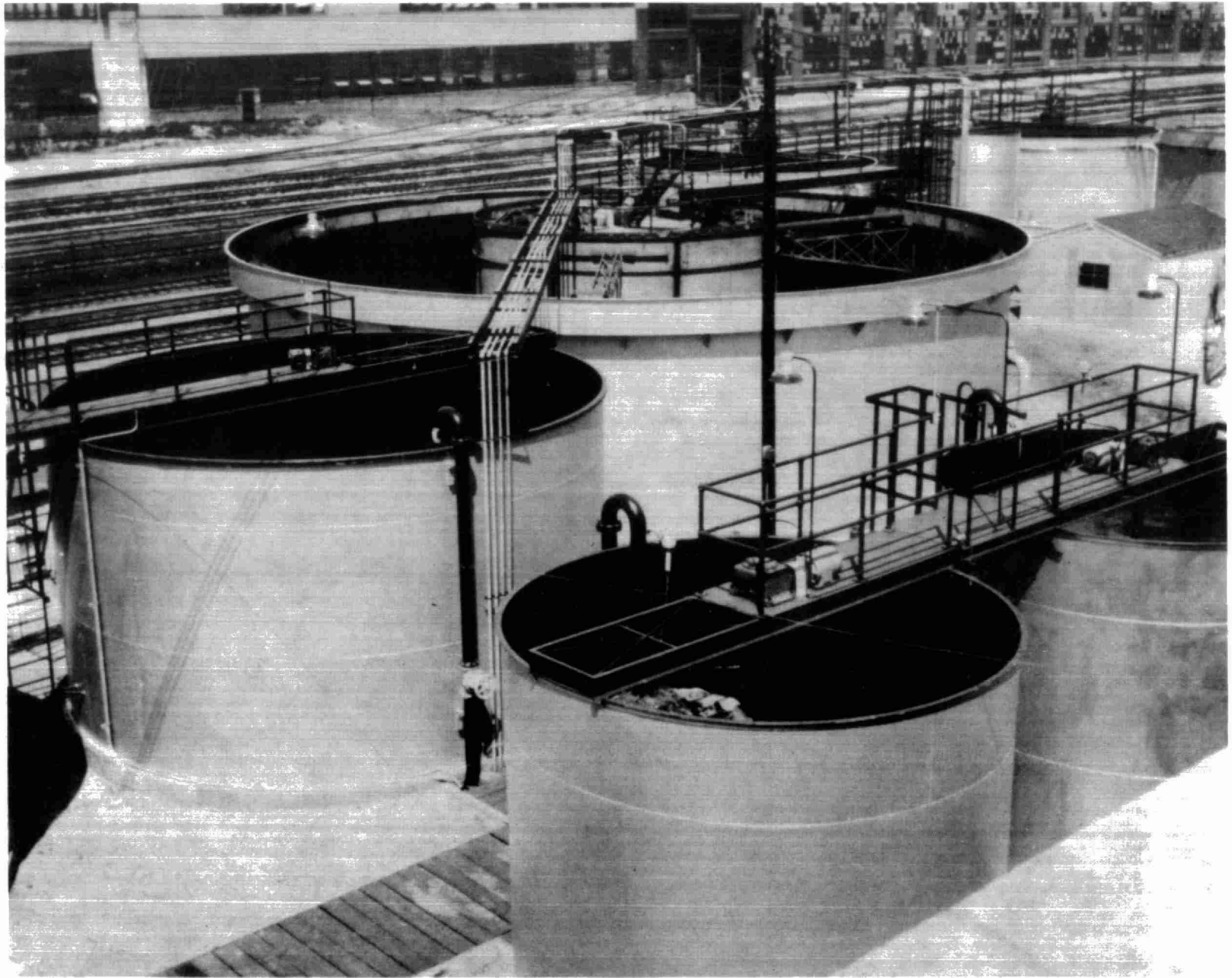
— FIGURE 11, INSTALLATION DETAILS OF TANKS IN THE TREATMENT SYSTEM SHOWN IN FIGURE 10 —
