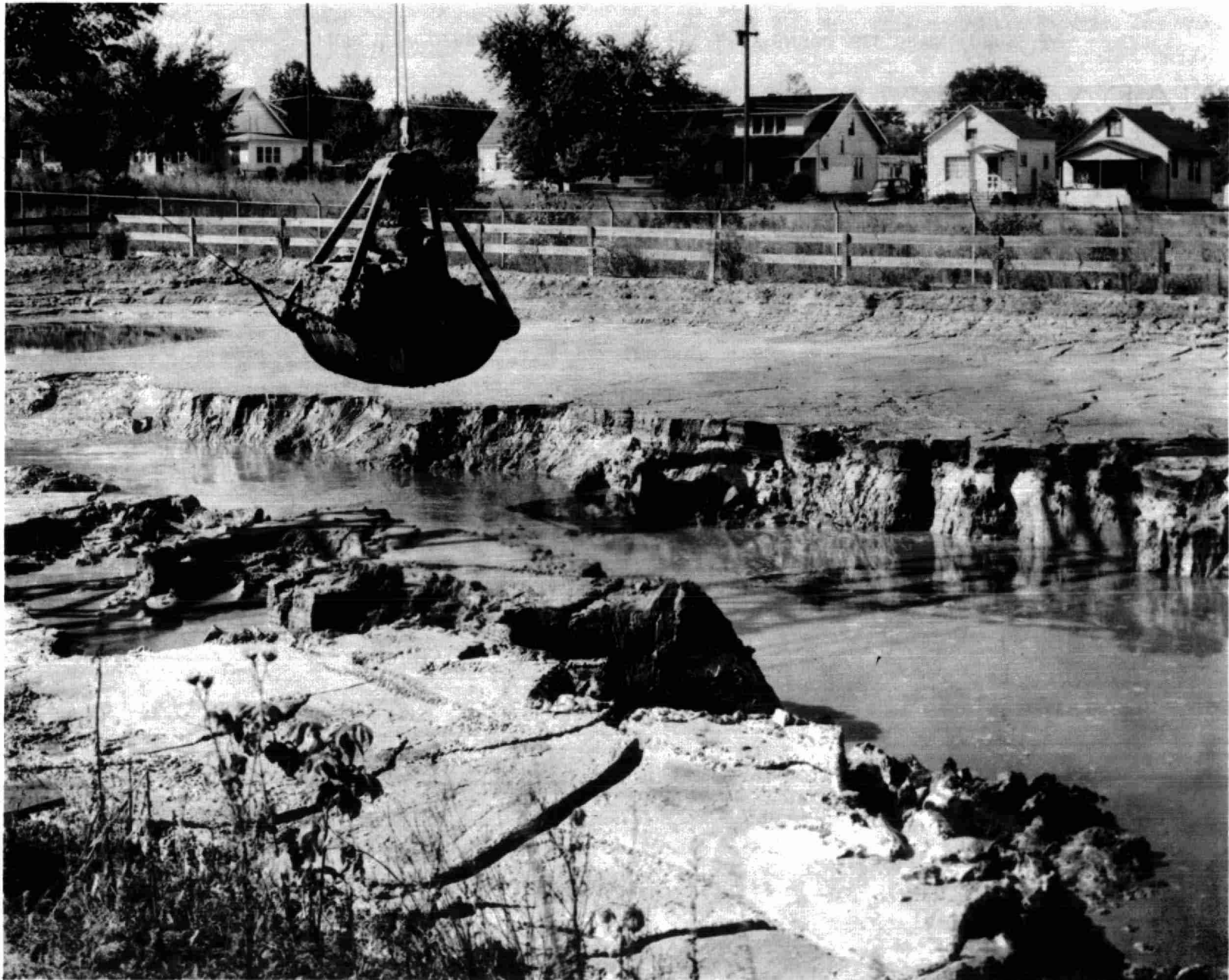
— FIGURE 14, APPEARANCE OF SLUDGE FROM PICKLE LIQUOR NEUTRALIZATION AFTER SEVERAL MONTHS OF DRYING —
