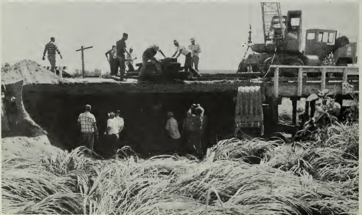
6. Storm runoff in August 1968 caused overflow adjacent to bridge on Highway 138 requiring extensive backfill to support concrete highway slab.
