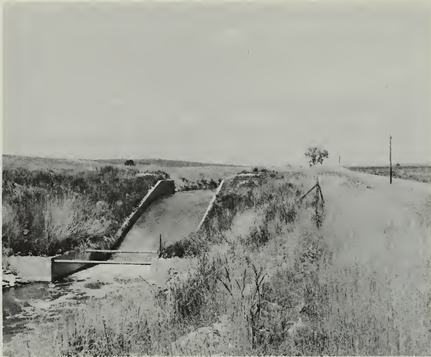
Looking northwest at drop structure in the Julesburg Irrigation District canal system. Canal delivers irrigation water to farms.
