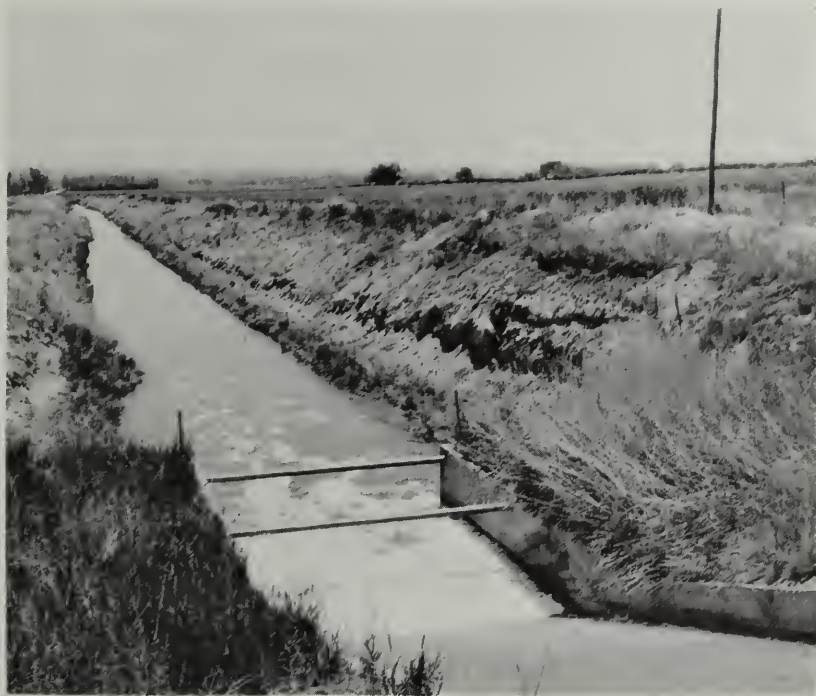
Part of the canal system of the Julesburg Irrigation District. Town of Sedgwick, Colorado, is in the background.
