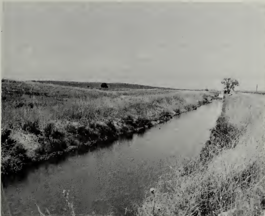
Floodwater and sediment from the upper watershed (left) enter the canal system causing sediment deposition in the canal and overtopping.
