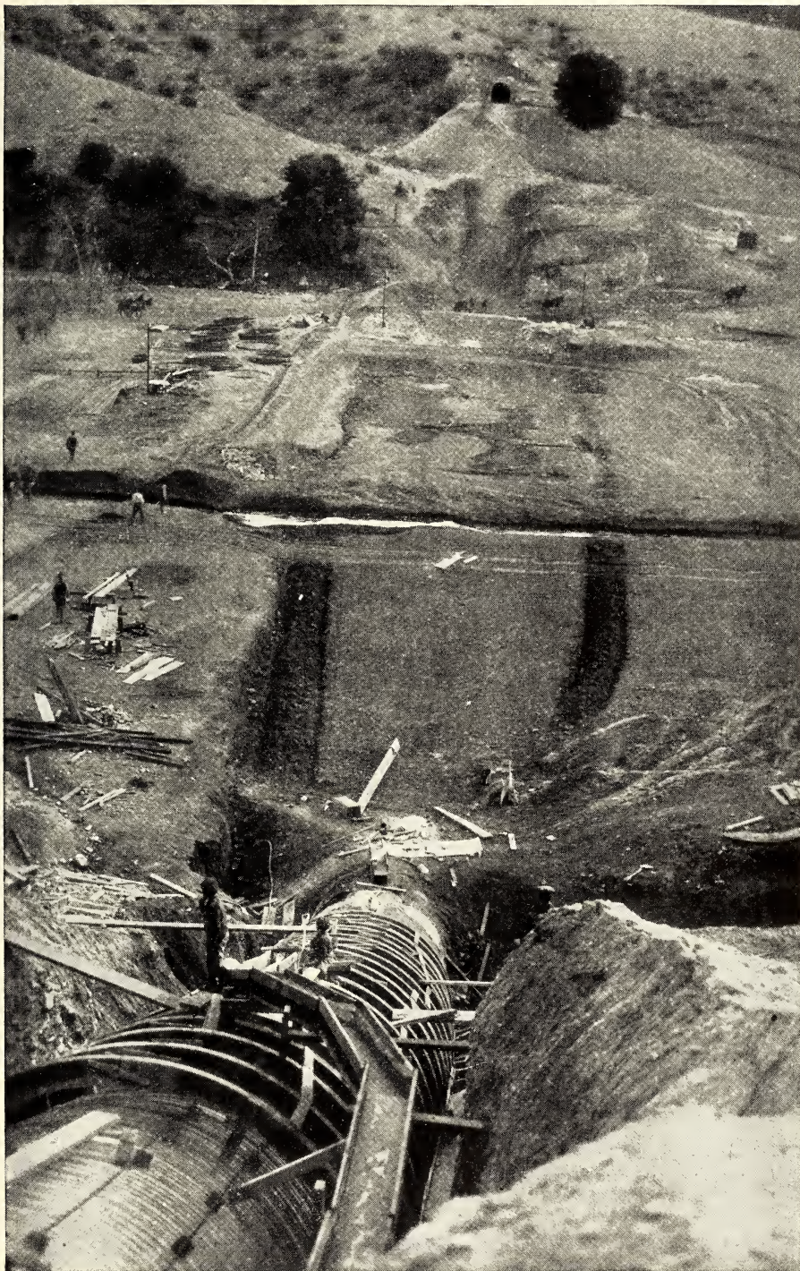
BUILDING AN INVERTED SIPHON ACROSS WHITNEY CANYON TO CARRY THE WATER DOWN ONE SIDE AND UP THE OTHER (SEE PAGE 574)
