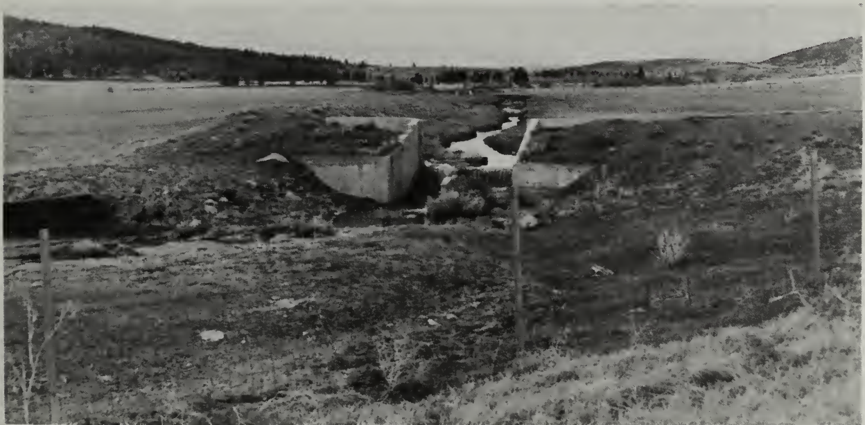
Water control structures such as this drop structure on Baxter Creek are important in the Calvada Subbasin.
