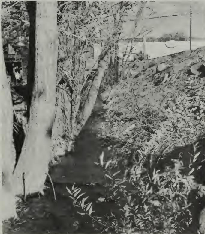
The Piute Creek flood channel through Susanville, Calvada Subbasin, will be protected by a floodwater detention structure above the city.
