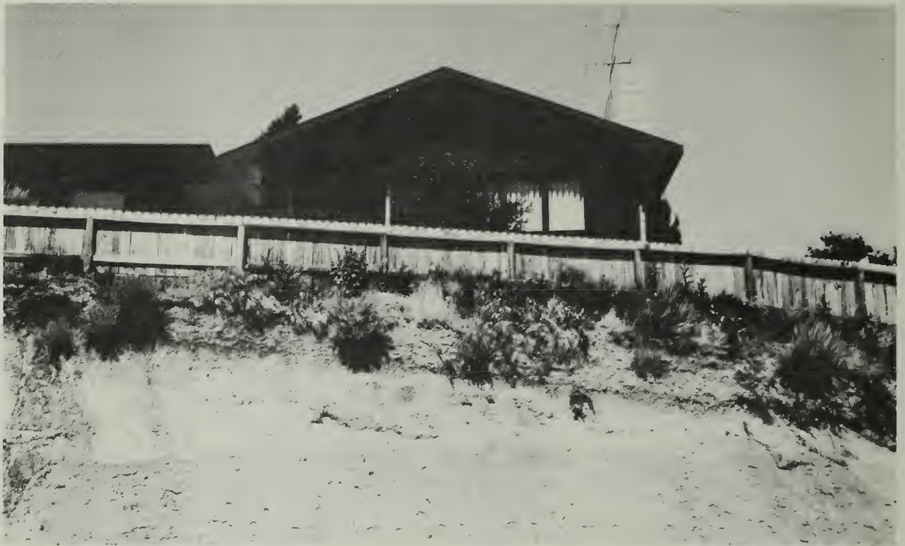
Southwest Reno. General Soil Map unit 30. Physical Land Use Suitability: grazing, rating good. Steep embankment is cut into soft bedrock creating erosion problem.
