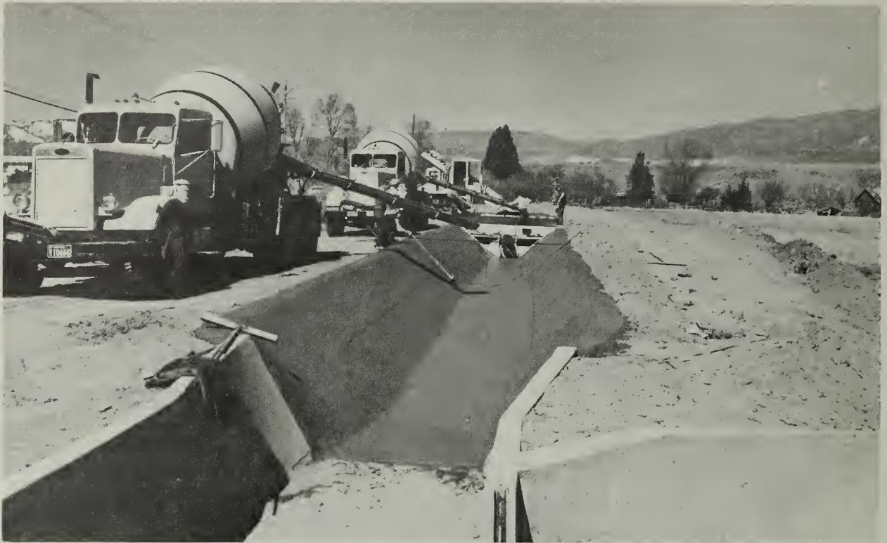
Concrete ditches (above) and sprinkler systems (below) will improve irrigation water use efficiency on the irrigated lands.
