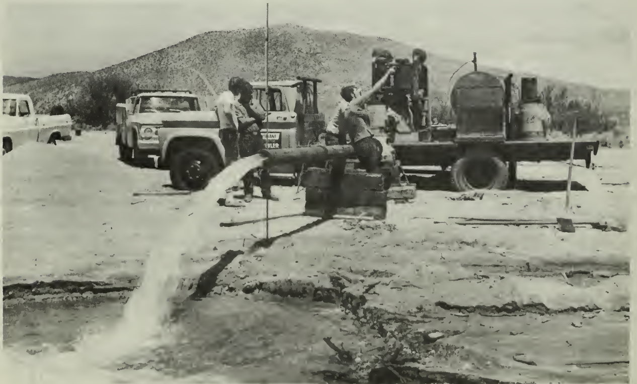
This well is being developed for municipal and industrial water for Carson City. Pat Glancy photo.
