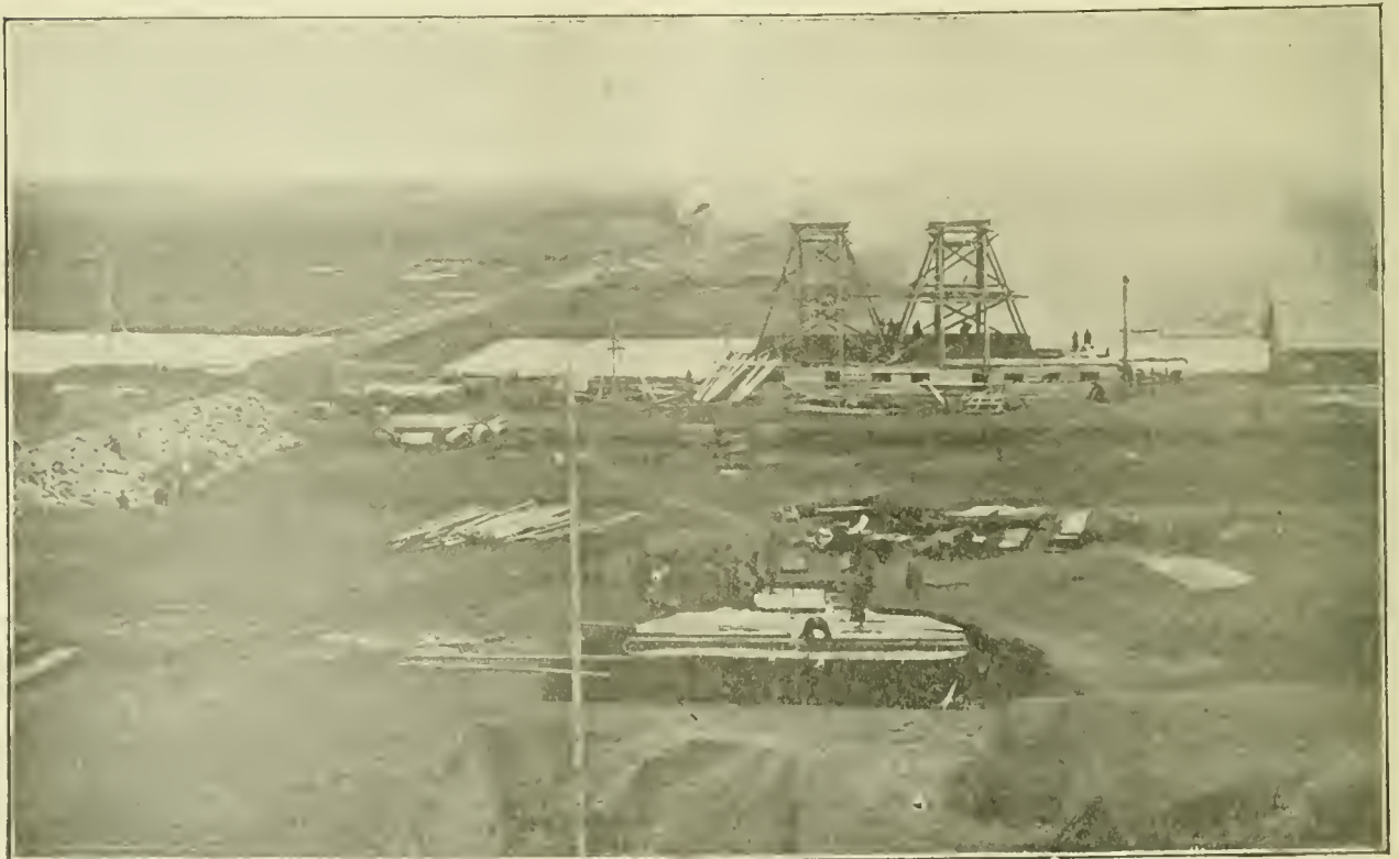
CONSTRUCTION OF THE ISHIM BRIDGE, SINKING OF THE FIRST CAISSON AND THE TEMPORARY BRIDGE.
