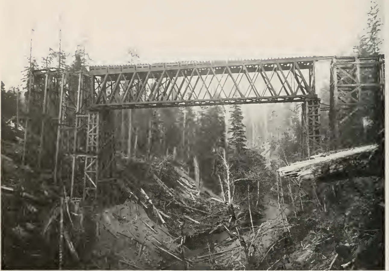
SIMPSON LOGGING CO.'S BRIDGE IN CONSTRUCTION STAGE. BEGINNING OF FOOT-HILLS OF THE OLYMPICS.
