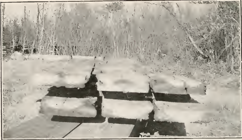
DECK PLAN REPLACED BECAUSE OF DECAY.
