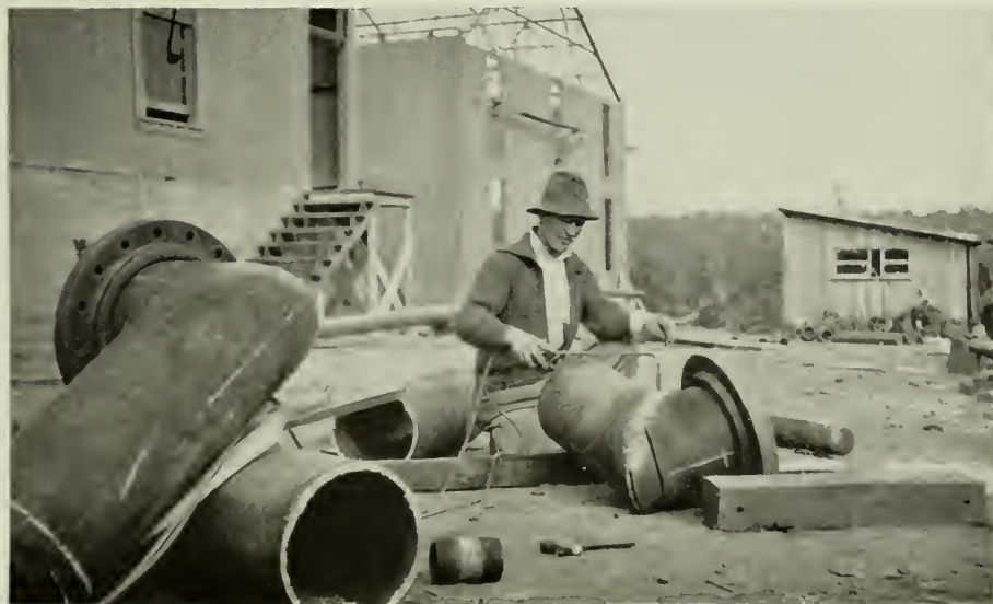
View showing how the natural gas man makes his own fittings in the field. Welding is rapidly taking the place of threaded joints and is far more leak-proof.
