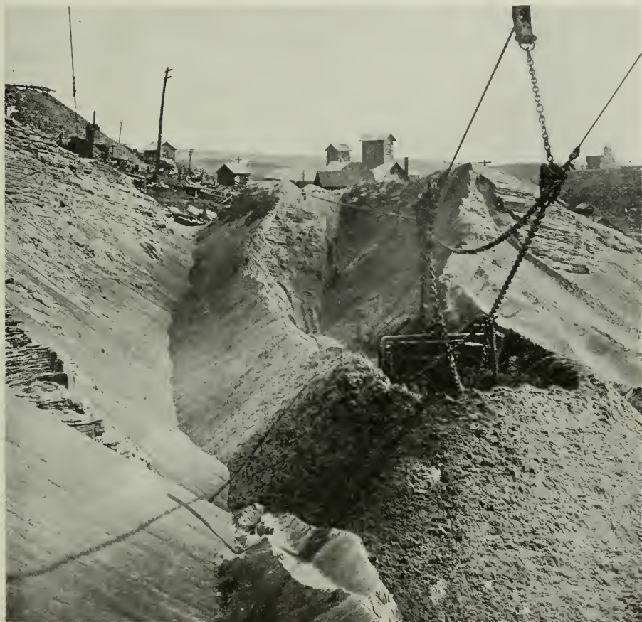
Sauerman drag-line excavator at Coniagas mine reclaiming sands carrying 3 to 3½ ounces of silver per ton. The sand is re-ground in tube mills to 100-mesh and treated by the flotation process.
