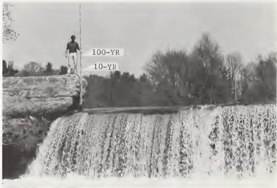
Sennebec Pond Dam, cross section 23D - The estimated level of the 100-year flood above this dam is 91.9 feet NGVD or 2.8 feet above the point where the person holding the board is standing. (SCS photo)
