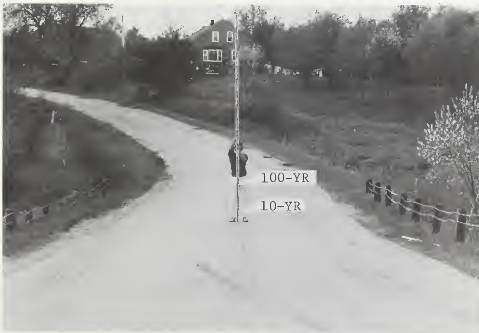
Medomak River, North Union Road, cross section M26C. The 100-year flood is estimated to be at elevation 181.8 feet NGVD or 2.9 feet above the road. This crossing has washed out on several occasions. (SCS photo)
