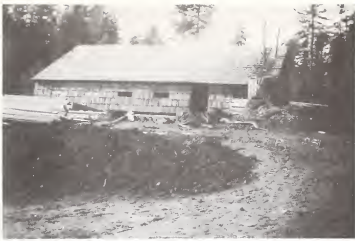
The mess hall at Camp Remote, Camas Valley, Oregon, during the latter stages of its construction at the time of our arrival.
