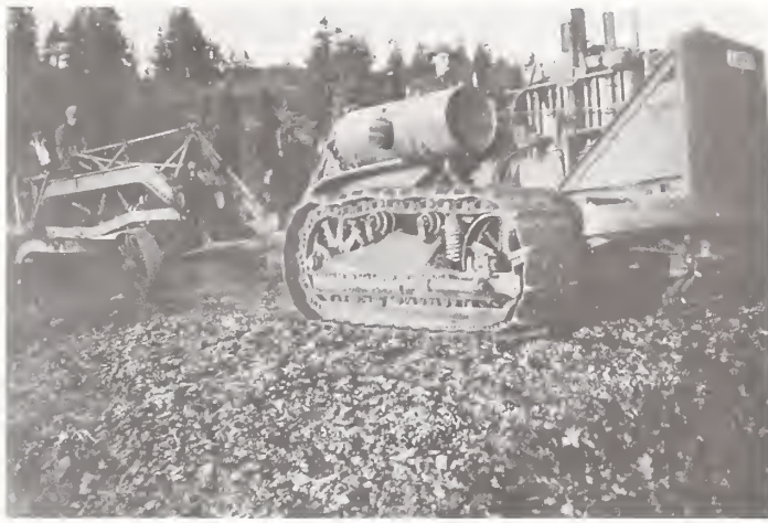
Albert Schloalman and Hank Anderson operating the caterpillar tractor and grader at Bald Ridges.
