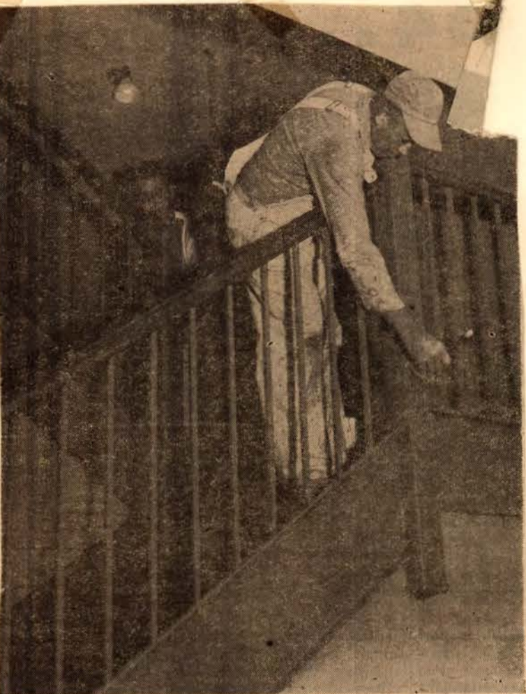
SPRUCING UP —Painters J. W. Banks, left, and J. T. Hawkins lean into their work at the Naval hospital here as they paint a ladder railing. The paint work is part of a several-months-long remodeling and renovation project carried on by the hospital's Maintenance department that has seen the clean-up paint-up work extended to all parts of the buildings and grounds at Hospital Point (Official USMC Photo).
