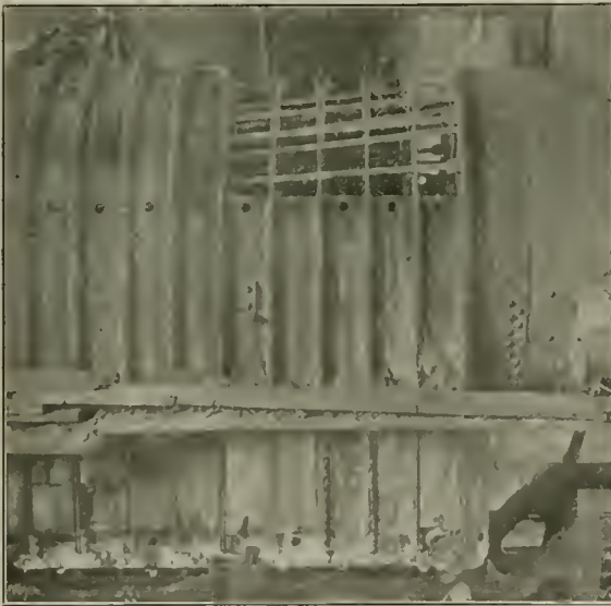
Fig 3—Defective Outside Top Sections Removed
