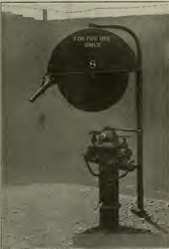
The Covered Reel Installed Near a Hydrant
