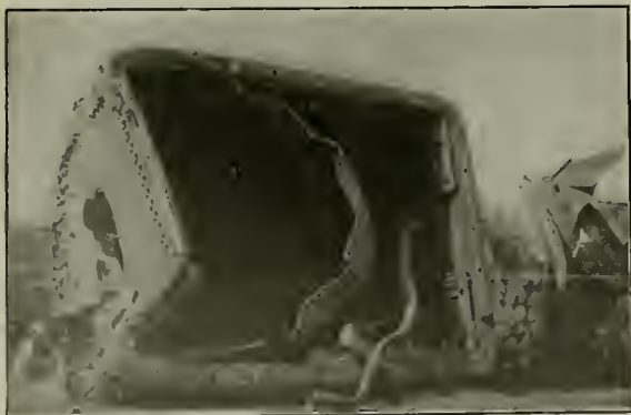
Dropped Crown Sheet Due to Low Water, Showing Failure of Welded Seam
