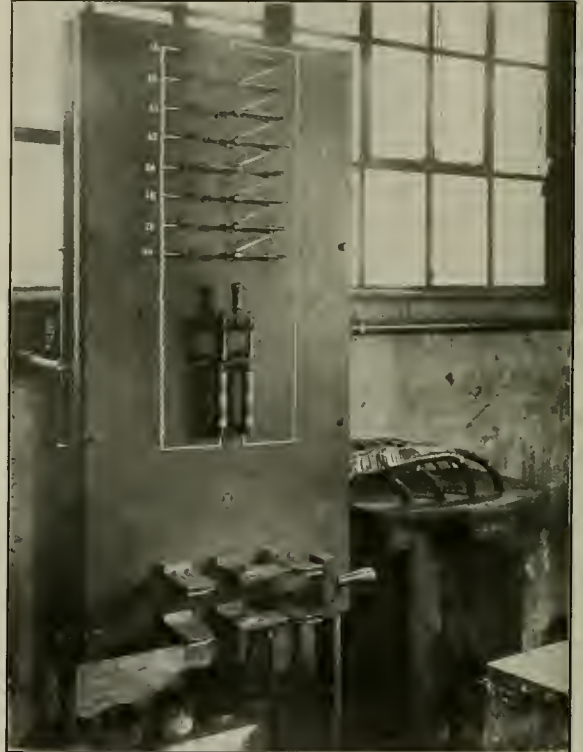
Switchboard and Transformer for Controlling Alternating Current Supply to the Tool Tempering Furnace
