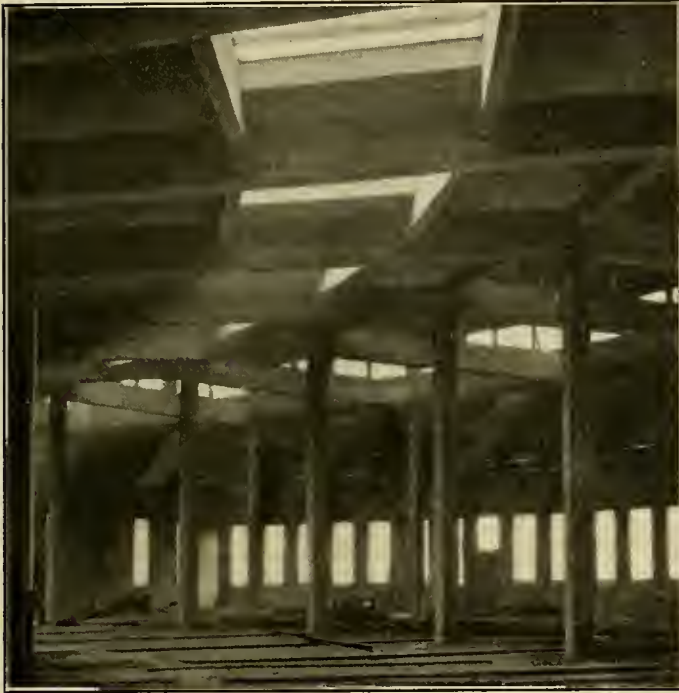
INTERIOR OF THE OAK HILL ENGINE HOUSE SHOWING SKYLIGHTS. (FLAT SKYLIGHTS ARE NOT USUALLY TO BE RECOMMENDED.)
