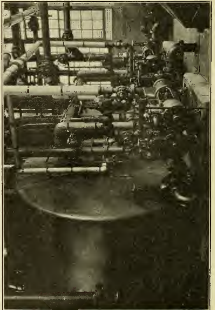
PUMPS, PART OF TANKS AND CONNECTIONS FOR THE HOT WATER WASHING AND FILLING SYSTEM
