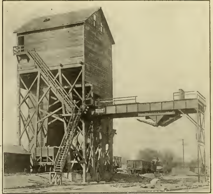
300 TON COALING STATION ERECTED BY FAIRBANKS, MORSE & CO., AT AUGUSTA, KAN. THIS STATION IS TYPICAL OF THE LARGE NUMBER ERECTED BY THIS COMPANY FOR THE SANTA FE AND IS PROVIDED WITH 10-TON AUXILIARY SCALE POCKETS, WHICH PERMIT THE ACCURATE WEIGHING OF THE COAL PUT ON EACH LOCOMOTIVE TENDER. THIS STATION COALS FOUR TRACKS AND OTHERS OF THE SAME TYPE WITHOUT THE BRIDGE COAL TWO TRACKS
