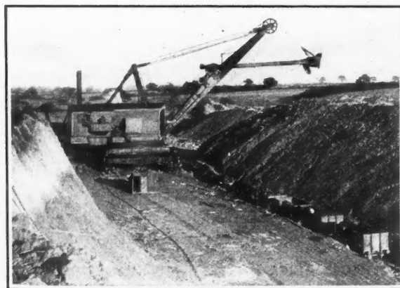
Fig. 2—Long-boom, full-circle steam shovel, of 7 cu.yd. capacity, installed recently by the Lloyds Ironstone Co.
