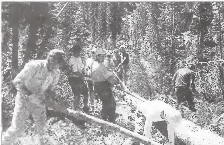
American Hiking Society volunteers move a log for bridge support on the Teton Creek Trail.
