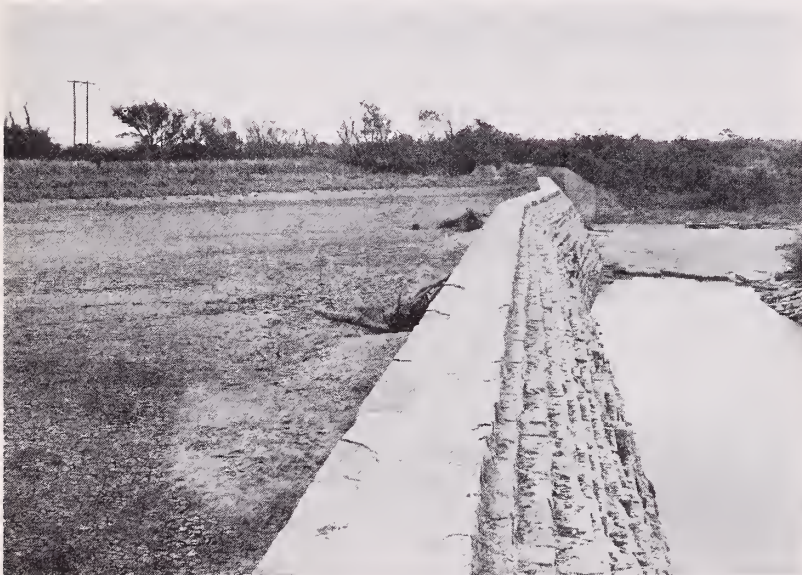
Soil from eroding farmland filled up this Texas lake which, at one time, was more than 35 feet deep. Proper land treatment would have prevented this siltation. TEX 48-840B
