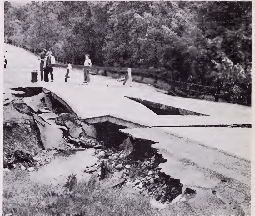
A stream swollen with an excess of runoff water undercut this section of a highway causing it to collapse. Floods also damage bridges and wash out country roads. CONN 10249
