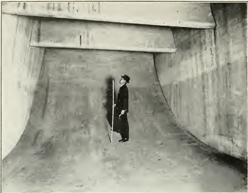
1. EAST BLOWER AIR DUCT
