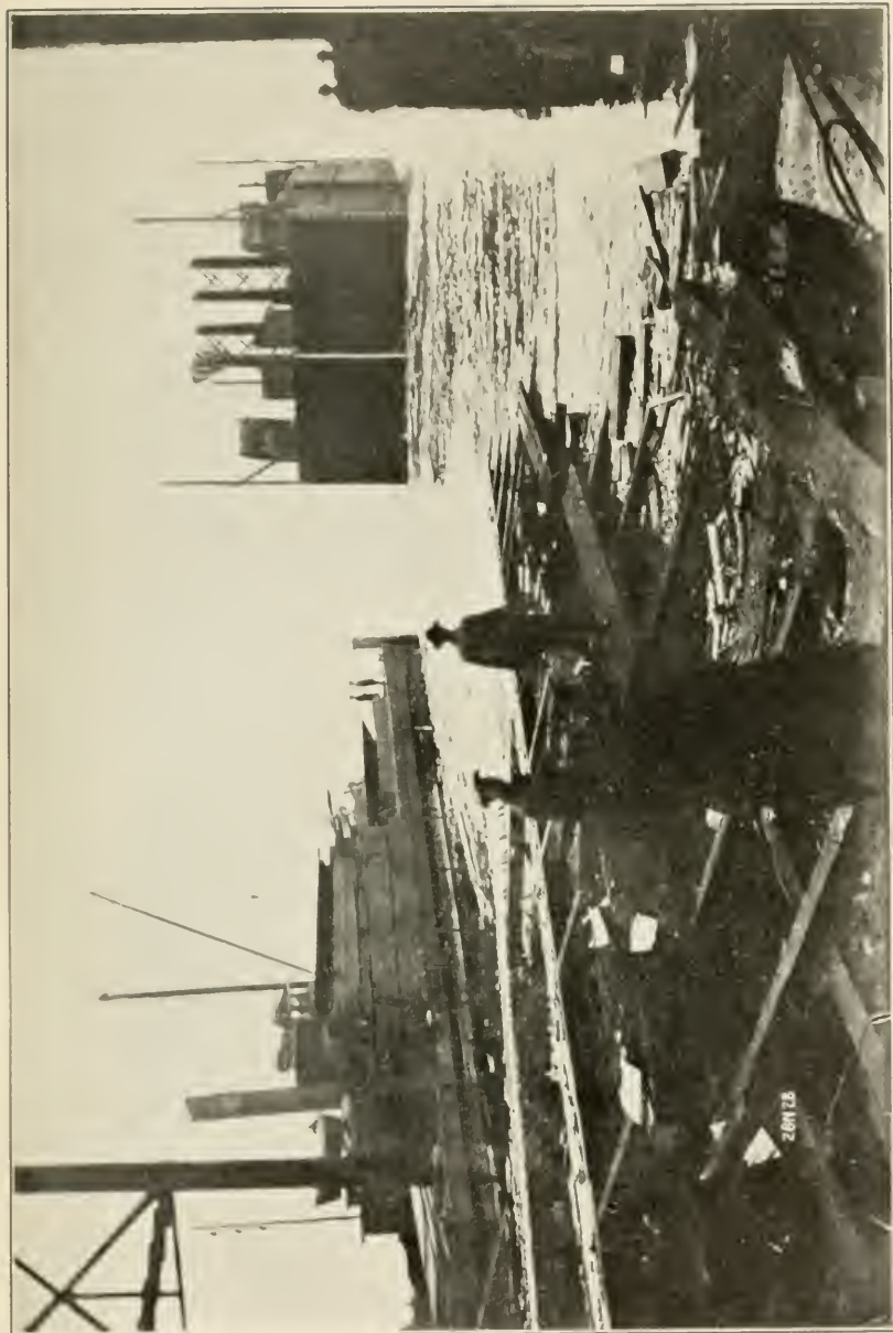
NEW JERSEY RIVER SHAFT CAISSON. JUST AFTER LEAVING THE WAYS Caisson launched at Mariners Harbor, Long Island, floated into position and sunk.
