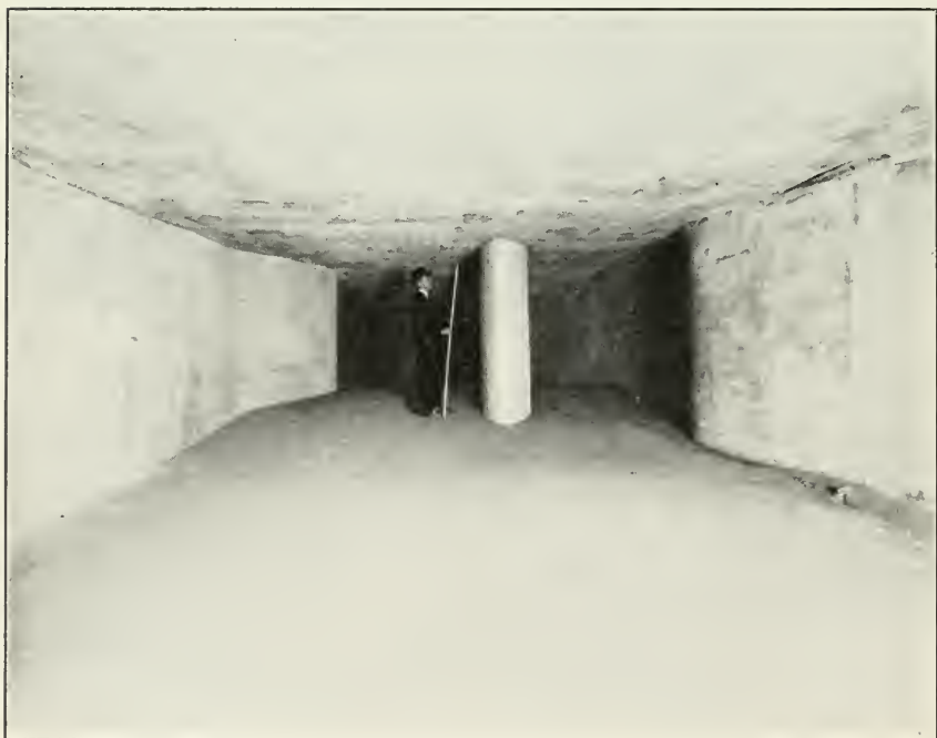
2. EAST BLOWER AIR DUCT
