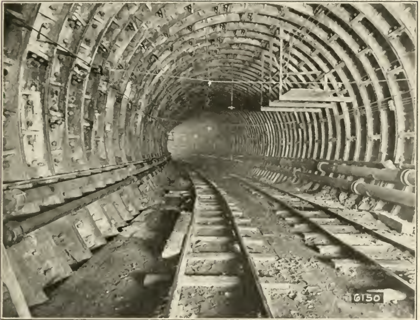
CURVE IN SOUTH TUNNEL UNDER WEST STREET, NEW YORK CITY (RADIUS 1,000 FEET). SHOWING COMPLETED RINGS OF CAST-IRON LINING
