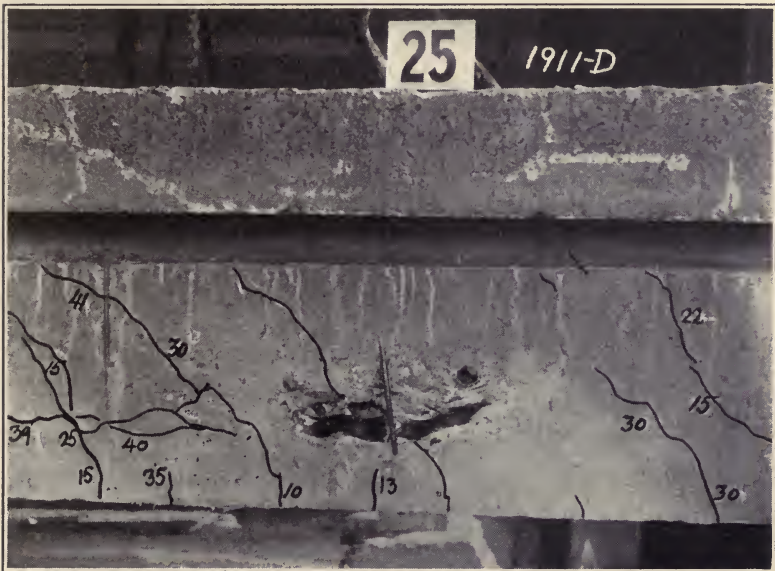
FIGURE 172. A CLOSER VIEW OF BEAM NO. 25, SHOWING CRUSHING OF THE CONCRETE AT THE ROD.
