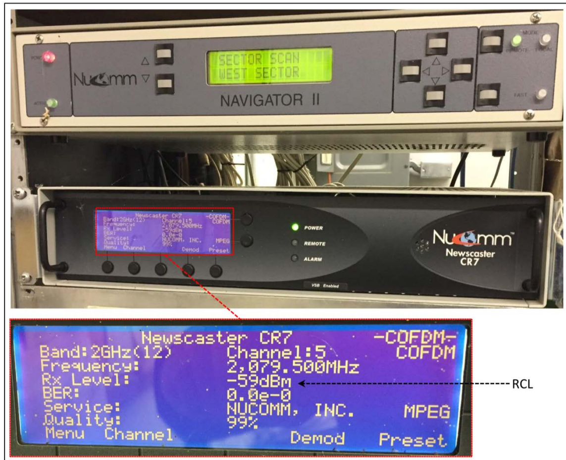
Figure 20. ENG Antenna Controller (NAVIGATOR II) and Receiver (NuComm Newcaster CR7). Source [25].
