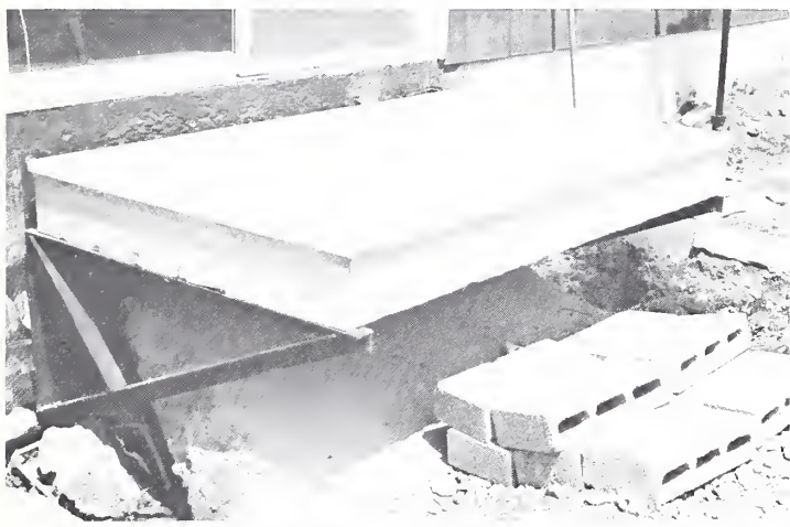
Back porch suspended—one of the many problems caused by sinking soil in the New Orleans area.
