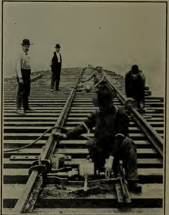
Fig. 197—Drilling rail-bonding holes. This shows the Williamsburg Bridge across the East River, between New York and Brooklyn, in course of construction.
