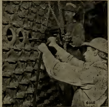
Fig. 87—Rolling boiler flues on a repair job with a Little David Pneumatic Drill.
