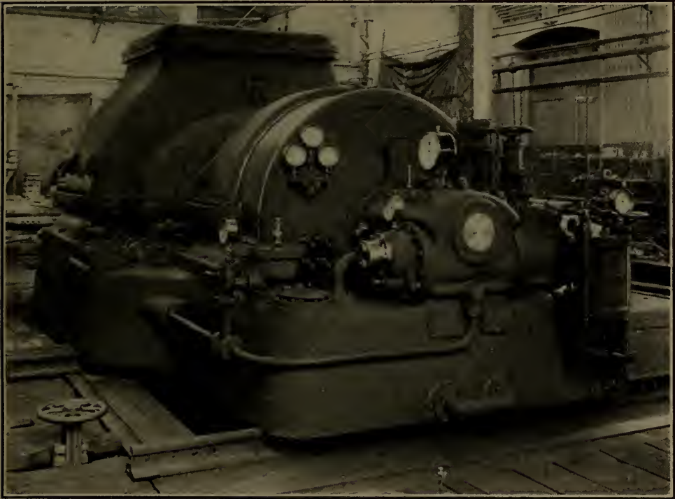
Fig. 21—Steam turbine-driven turbo blower.
