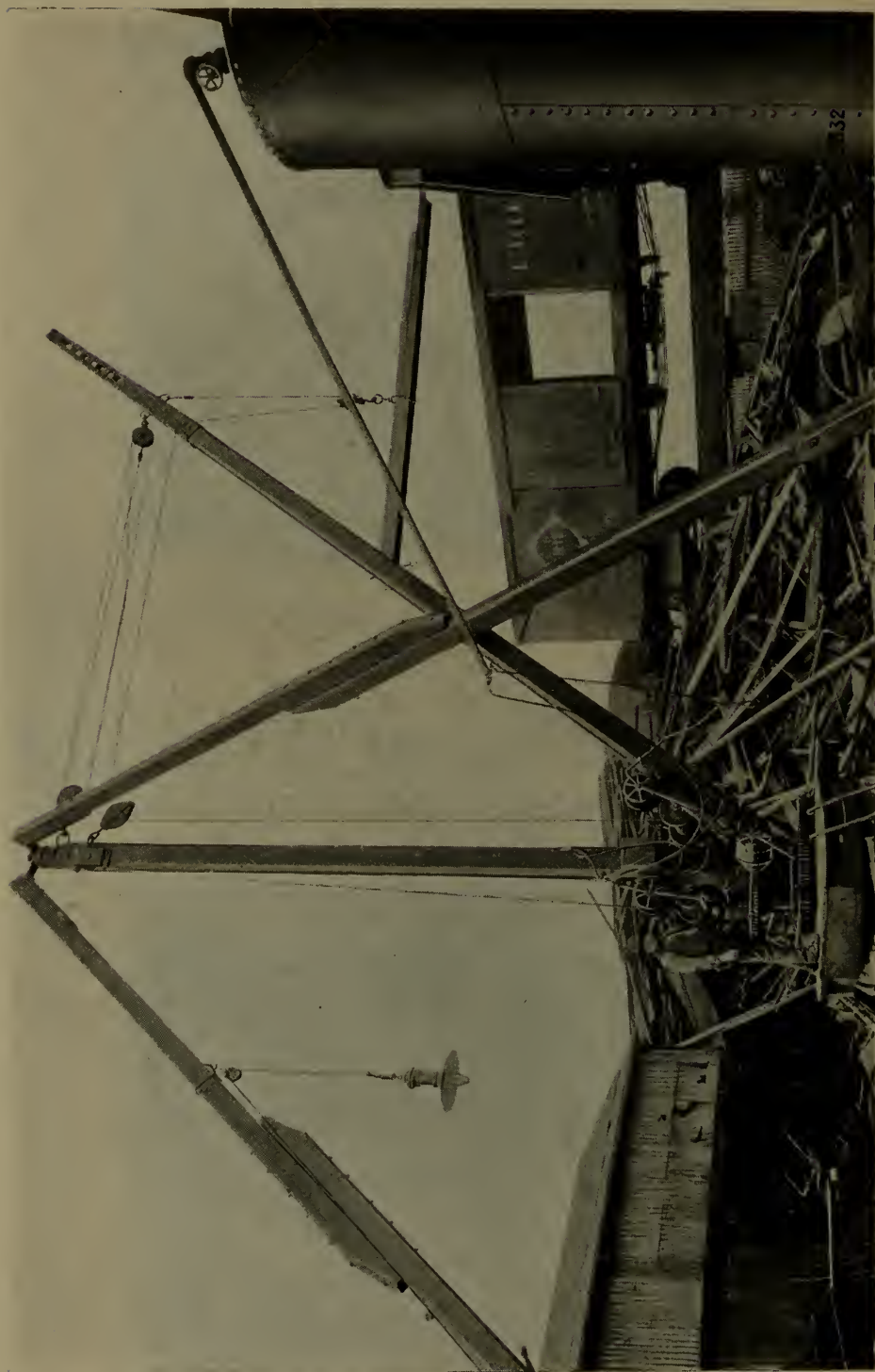
Fig. 236—Compressed air motor operated derrick in yard of the American Iron & Steel Co., Lebanon, Pa.
