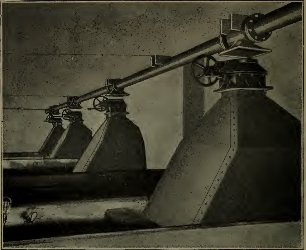
Fig. 251—Ash Conveying line and storage hoppers.
