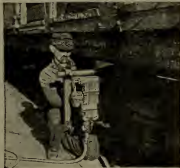
Fig. 200—Close quarter drill at work in the Middletown, N. Y., Car Repair Shop of the New York, Ontario and Western R. R.
