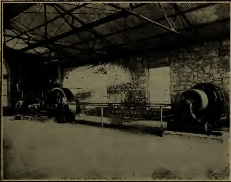
Fig. 1—The 'long-belted' type of air compressor drive. This shows a duplex two-stage machine.
