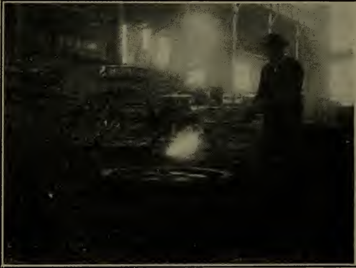
Fig. 123—Skin drying a gear wheel mold, 4 ft. in diameter to a uniform depth of \frac{1}{2} in. in 12 minutes with a Hauck Portable Oil Torch operated by compressed air.
