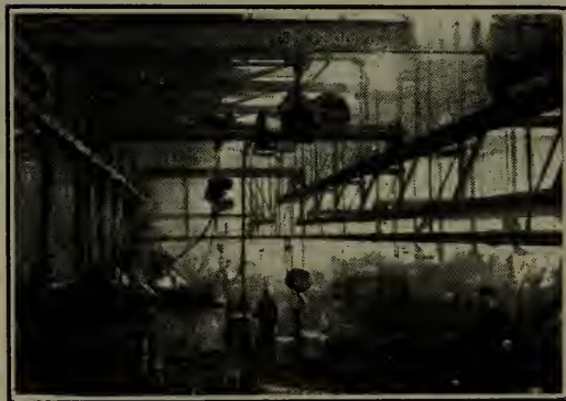
Fig. 117—In the foundry of McNab & Harlin, Paterson, N. J., a number of air motor hoists operating in conjunction with hand operated travelers meet all the requirements for hoisting and handling molds, patterns, cores, etc.
