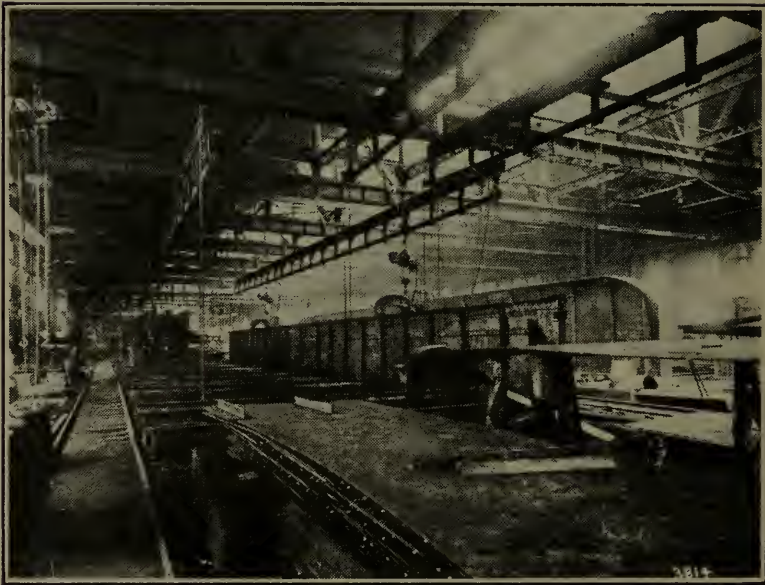
Fig. 218—Imperial Pneumatic Hoists and Pneumatic Yoke Riveter used in combination for fabricating structural steel shapes in the Lassig Plant of the American Bridge Co., Chicago, Ill.
