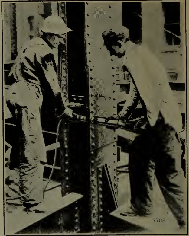
Fig. 211—This illustration shows the application of the pneumatic holder-on in riveting work.
