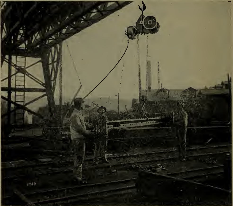
Fig. 243—An air motor hoist in the yard of a structural steel plant.
