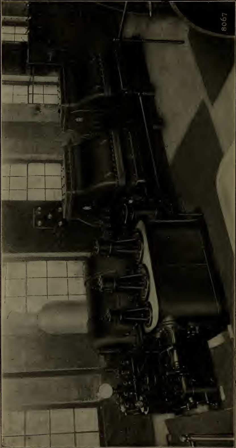
Fig. 20—Steam turbine-driven turbo air compressor.
