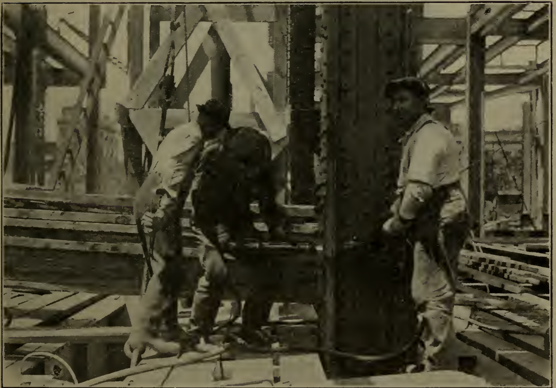
Fig. 214—Pneumatic riveter and pneumatic holder-on at work on new Public Service Building, Newark, N. J. Notice the TEE connection in the hose line for feeding air to both tools by means of one main hose line.
