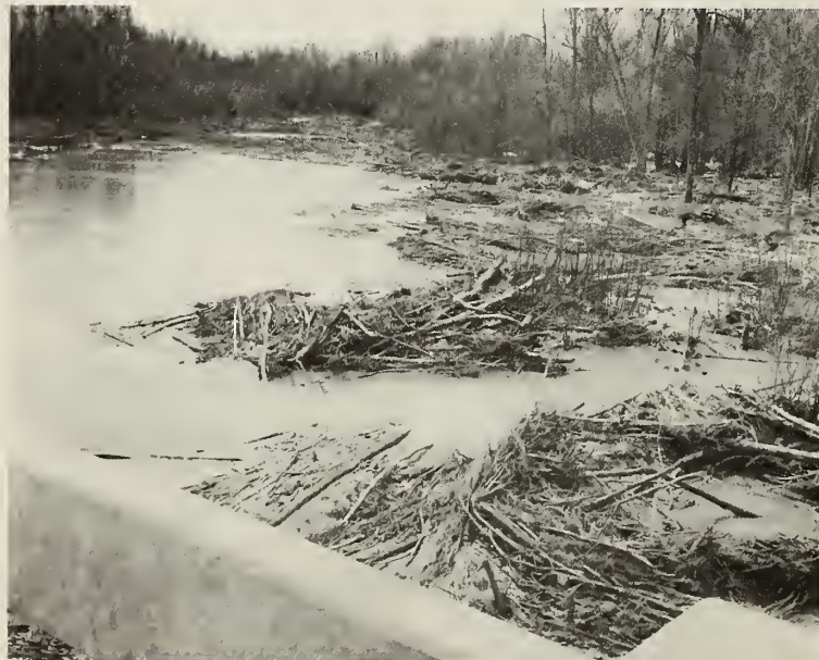
West side of bridge over Loosahatchie River on the Raleigh-Millington Road. Note log jams and other debris.
