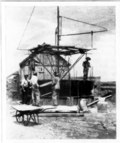
Mast and Movable Forms Which Speed Building of Circular Storage Bins of Reinforced Concrete
