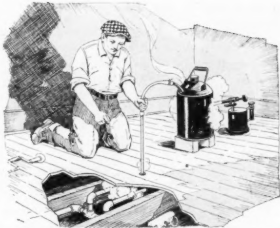
Frozen Water Pipes Thawed Out by Steam Admitted through Small Hole Drilled in Floor
