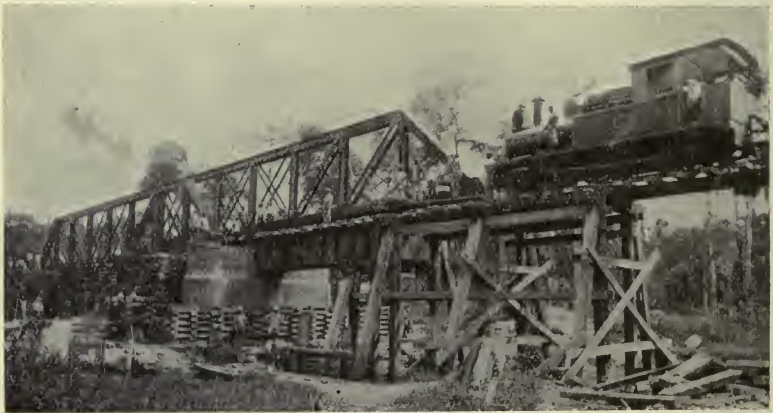
ENGINE PUSHING A GIRDER INTO POSITION OVER THE SAYONG RIVER (Johore State Railways)
