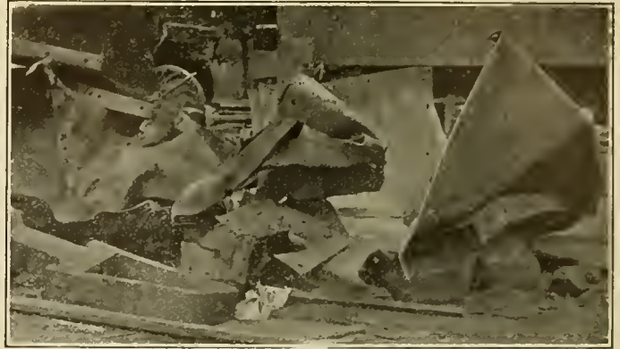
FIG. 31.—BADLY DAMAGED END SILL AND SHEETS.
