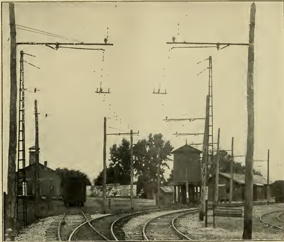
VIEW SHOWING BRACKET AND SPAN CATENARY TROLLEY SUPPORTS—ERIE ELECTRIFICATION.
