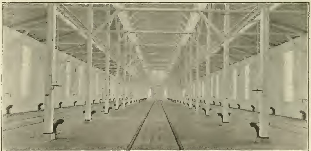
INTERIOR OF PAINT SHOP SHOWING HEATER PIPES.
